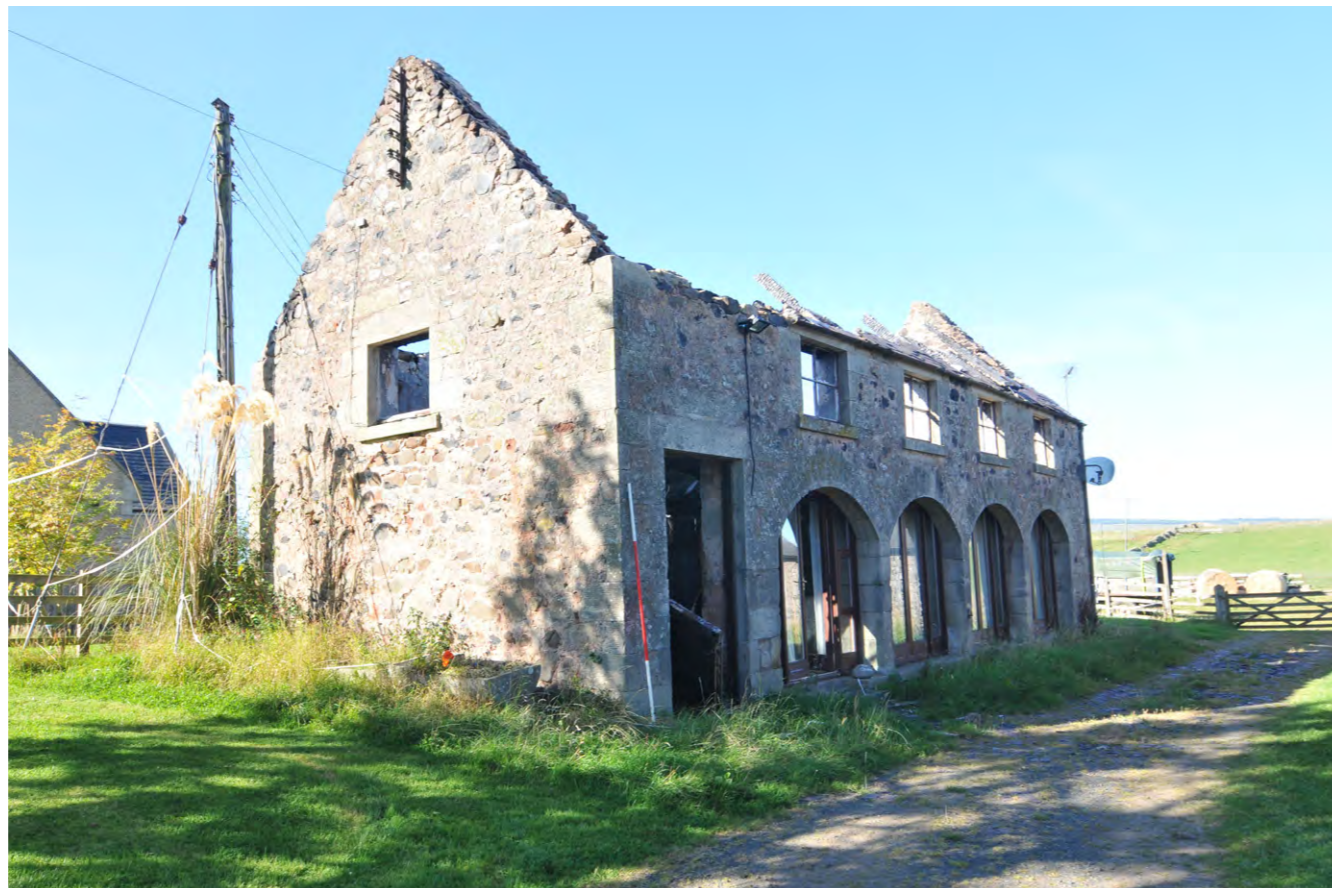
Fig. 24 General view of the fire-damaged former granary building and cart shed
