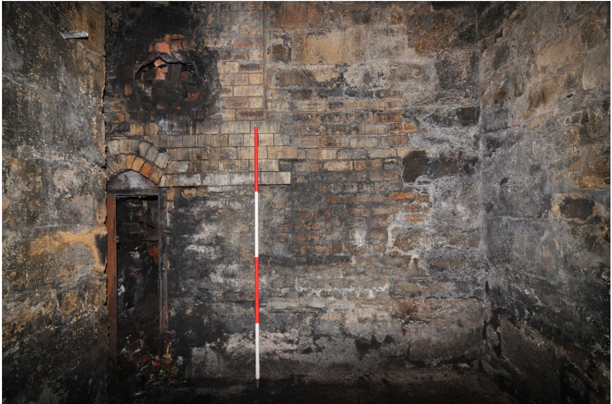
Fig. 13 - Interior east-facing elevation showing the chimney base and cast-iron door and wall faced with refractory brick
