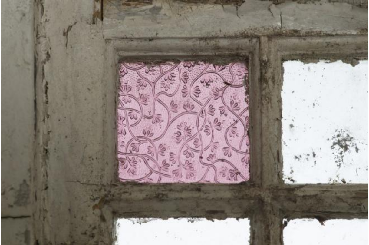
South Block, ground floor, entrance porch (0.20), detail of coloured glass (RCAHMS: DP194646)
