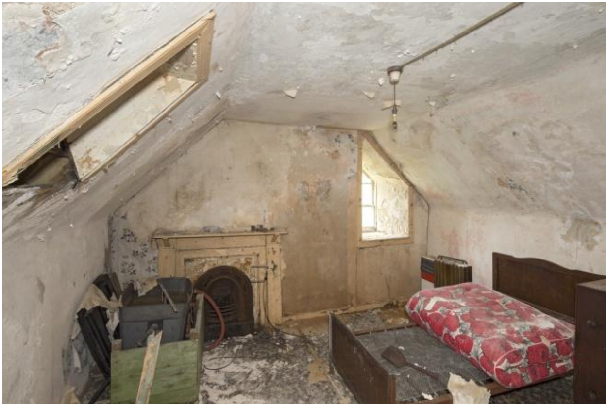
North Block, first floor, north bedroom (1.4), view from south west (RCAHMS: DP194669)
