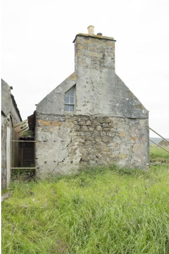
North range, east gable, view from north east showing narrow gap and link (RCAHMS: DP194627)
