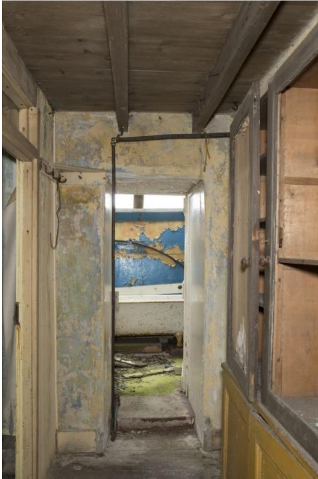
North west range, ground floor, corridor (0.2) to bathroom (0.3), view from south east (RCAHMS: DP194661)
