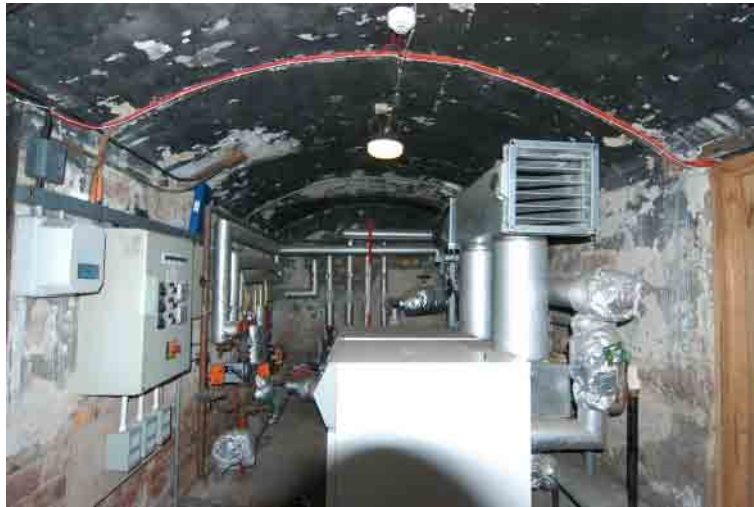
Fig. 16 Interior view of the basement boiler room with vaulted ceiling
