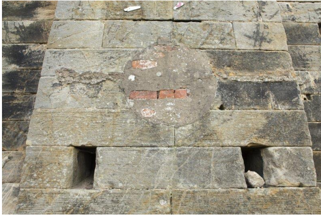
Above: View of base of west gable or 'bob wall' from west showing the buttress and the two slots in the wall fabric. These do not go right through the wall, but allowed access to the bolts which anchored the bearing on which the engine beam would have pivoted. The brick blocked aperture above is probably the waste steam pipe outlet which may or may not have connected with an external condenser box. [DP23201, HES]
