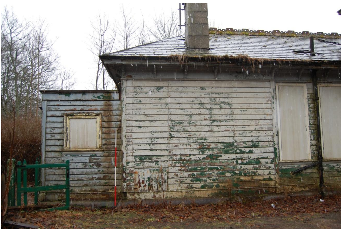
III 6 The extension on to the east end of the station building
