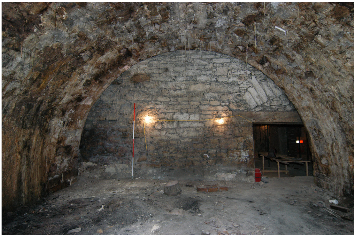
Fig. 7 Interior east-facing elevation of Vault 2 showing part of the larger opening with a segmented relieving arch
