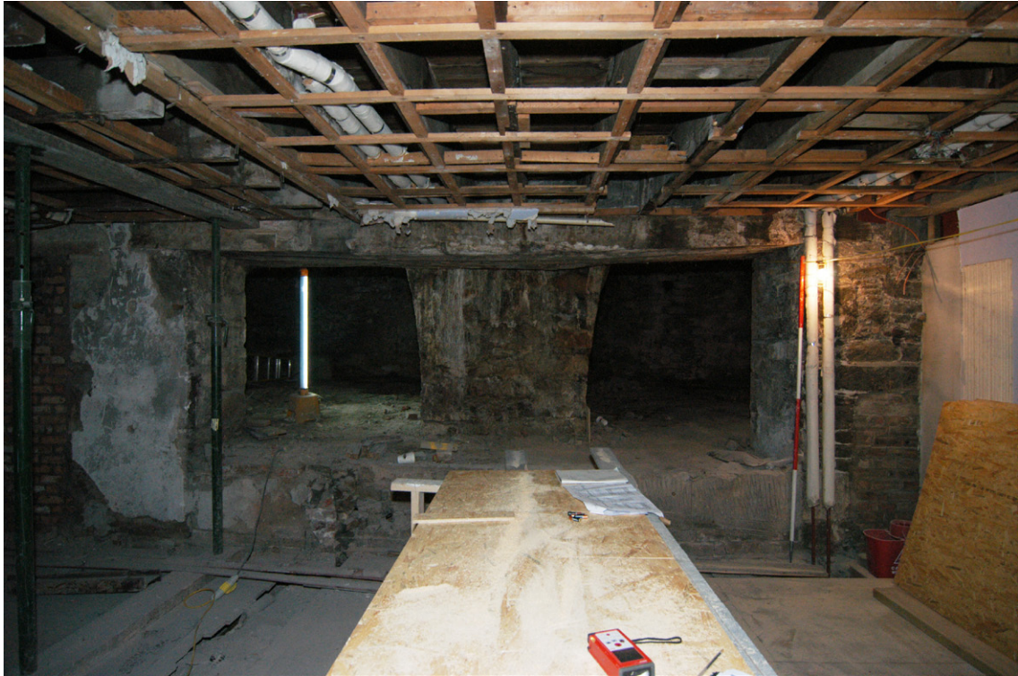
Fig. 8 Looking into Vaults 1 and 2 from within the main block of 85-87 South Bridge
