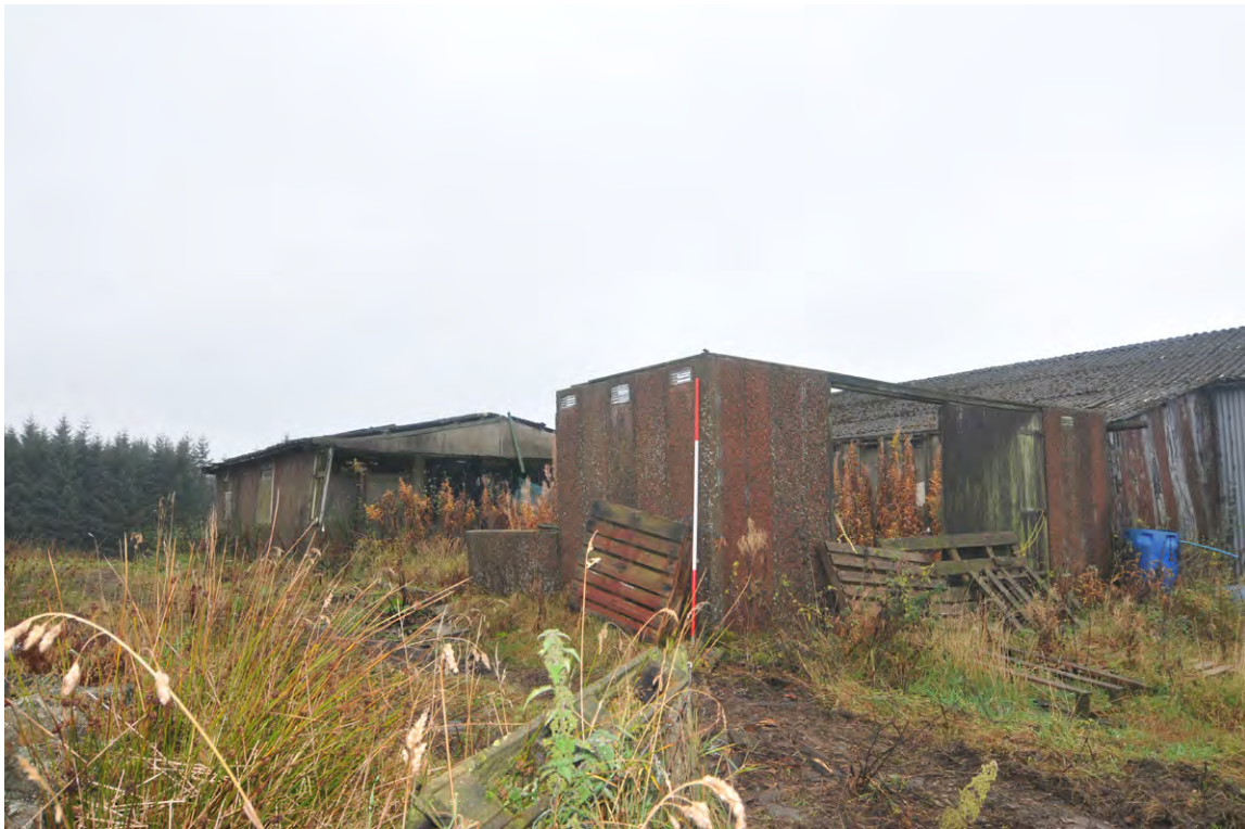
Fig. 21 Unit 17, derelict concrete shed, east-facing elevation
