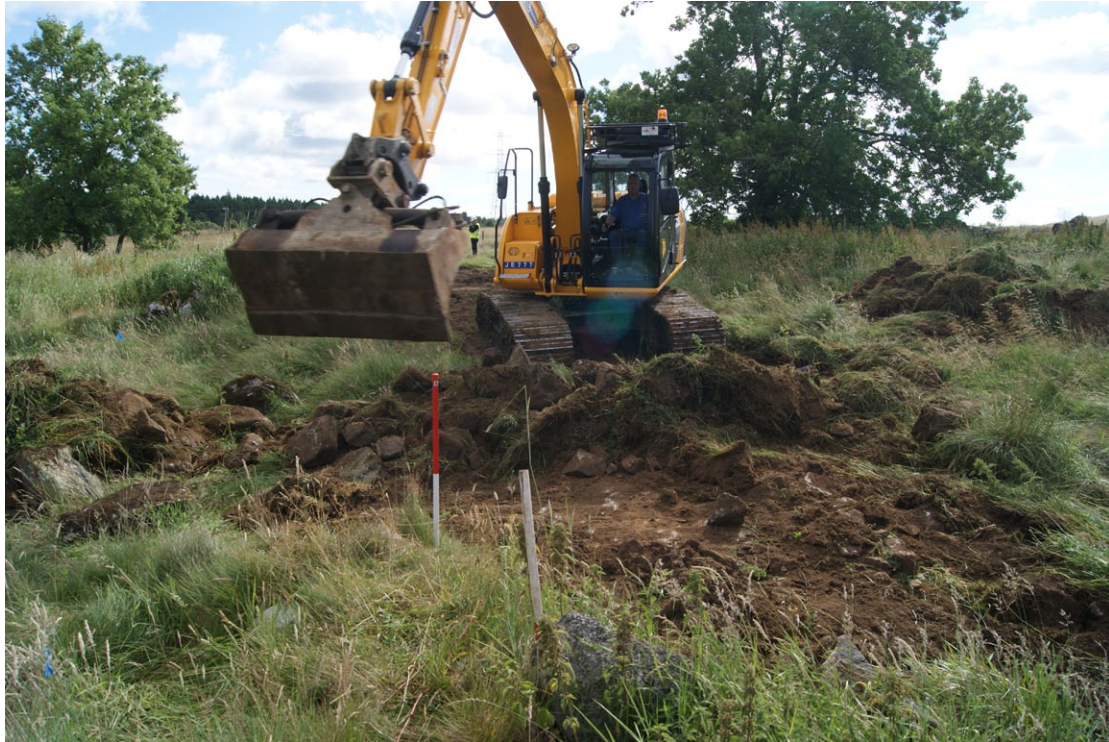
Fig. 19 - Supervising removal of boulders recently dumped against building 007, Queels
