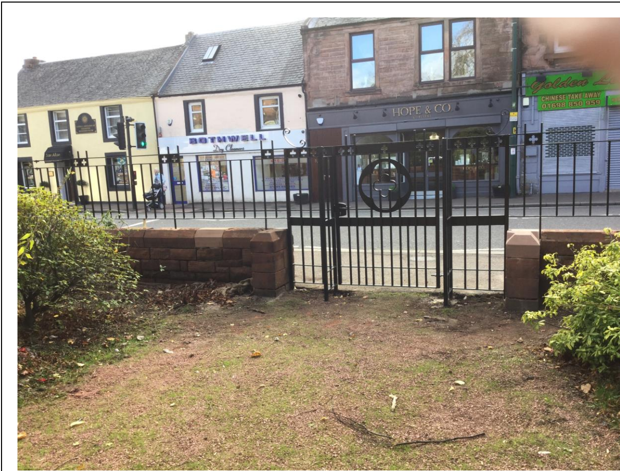
Illus.23 (6.3a/6.3f) Restored gateway at Dixon Gate, incorporating quatrefoil design, matching gate leading to old Manse. New gates have reduced the width of gateway.
