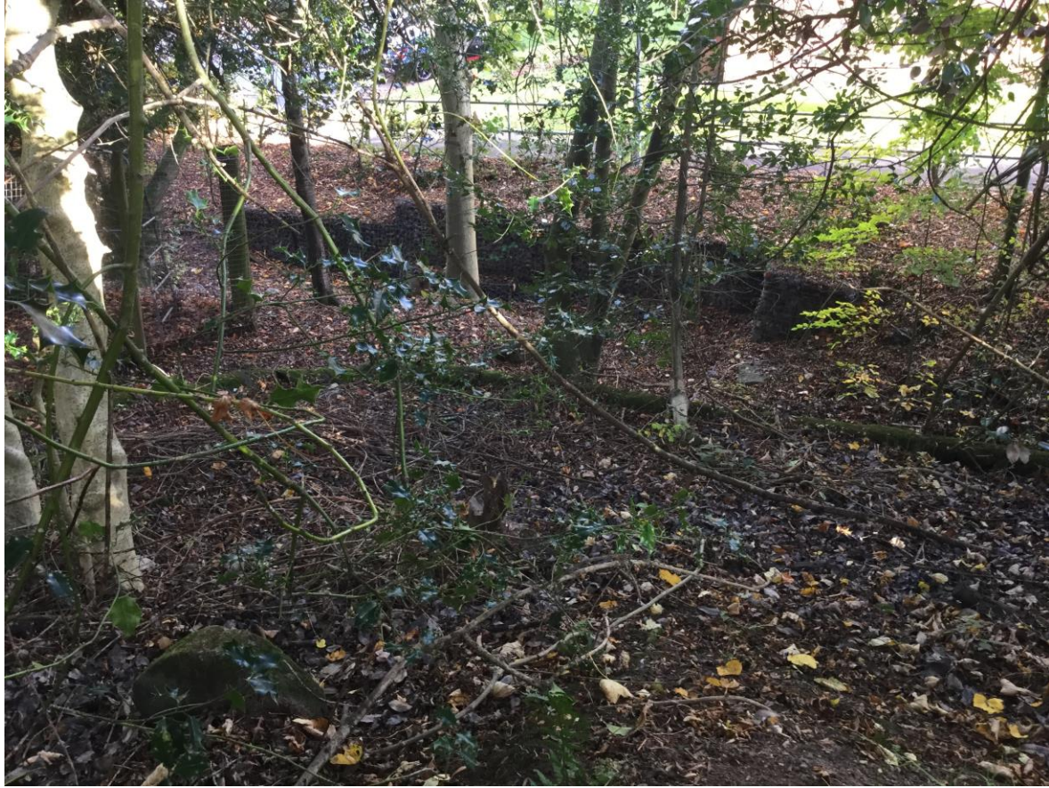
Illus.14 (6.2a) Boundary wall at NE section of graveyard slopes away to a 20 foot drop where only visible part of wall is coping stones. Retaining wall is also visible on opposite side of path running alongside boundary wall.
