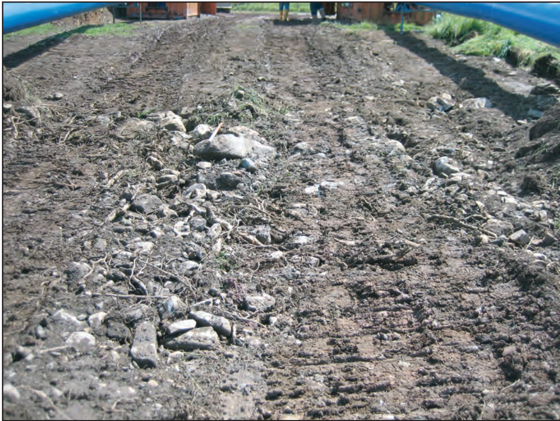
Plate 1: Rubble stone along the Shennanton to Ardachie pipeline corridor from the west
