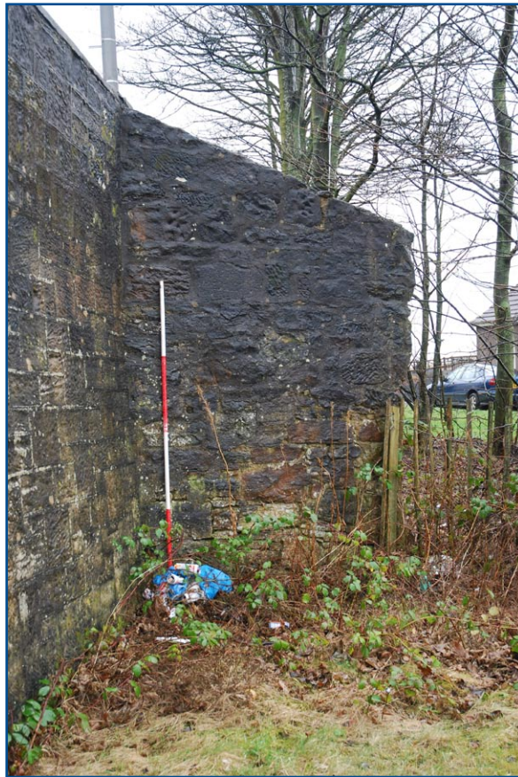
Plate 29: Detail of the stretch of wall on southern side of eastern wall to Maryhill Road
