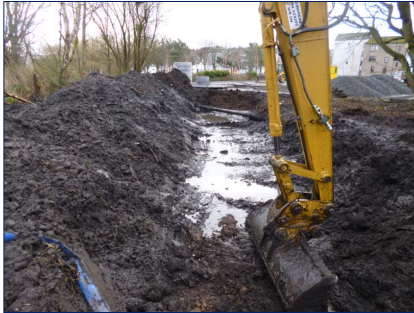
Plate 2- Excavation of Filter Trench to north of car park, with Sam's Dyke [012] in distance to east
