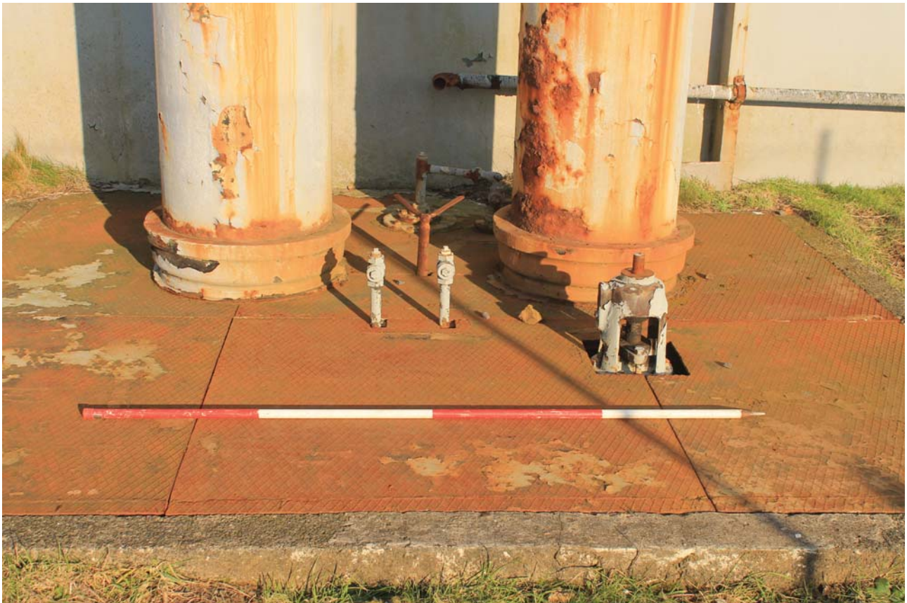
Plate 12: Weir Road, Newtown-on-Ayr, detail of pipe fittings on the pipes on the SSW side of the gasholder from the SSW
