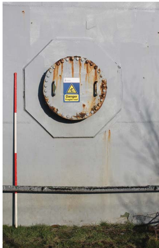
Plate 14: Weir Road, Newtown-on-Ayr, detail of inlet pipe on the south side of the gasholder from the south
