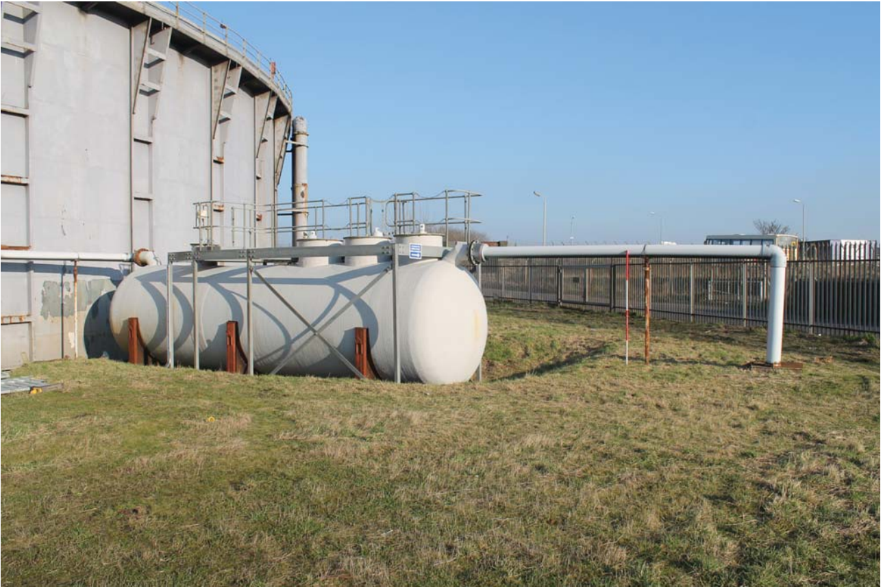
Plate 19: Weir Road, Newtown-on-Ayr, general view of the interceptor tank from the south-west
