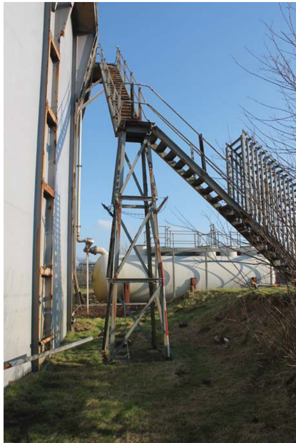
Plate 8: Weir Road, Newtown-on-Ayr, general view of the side of the stair from the south-west
