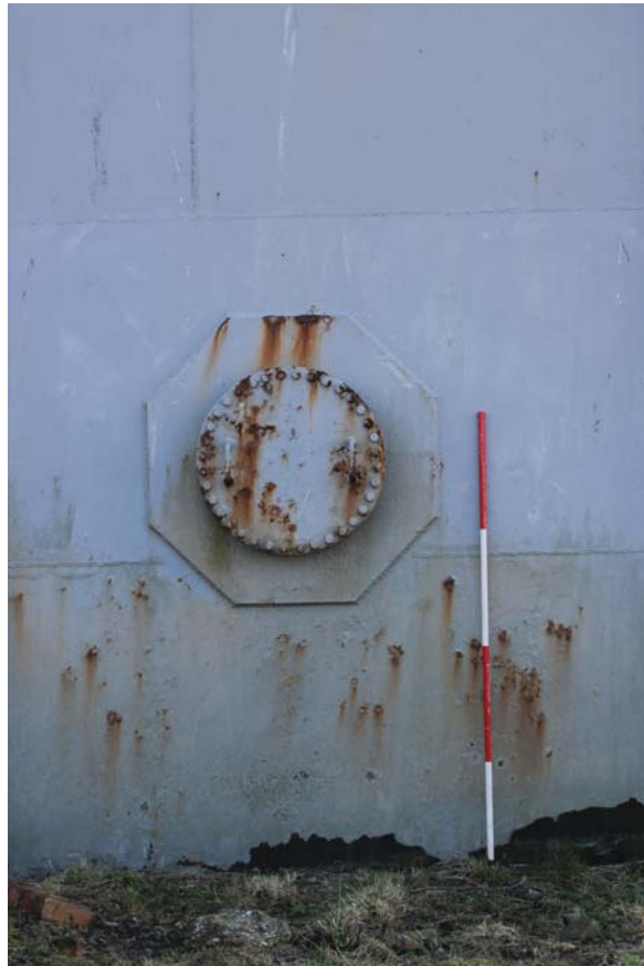
Plate 15: Weir Road, Newtown-on-Ayr, detail of the inlet pipe on the north-west side of the gasholder from the north-west
