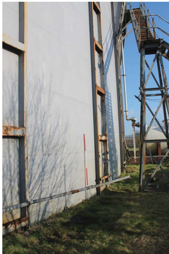
Plate 6: Weir Road, Newtown-on-Ayr, detail of stanchion on the south side of the gasholder from the west
