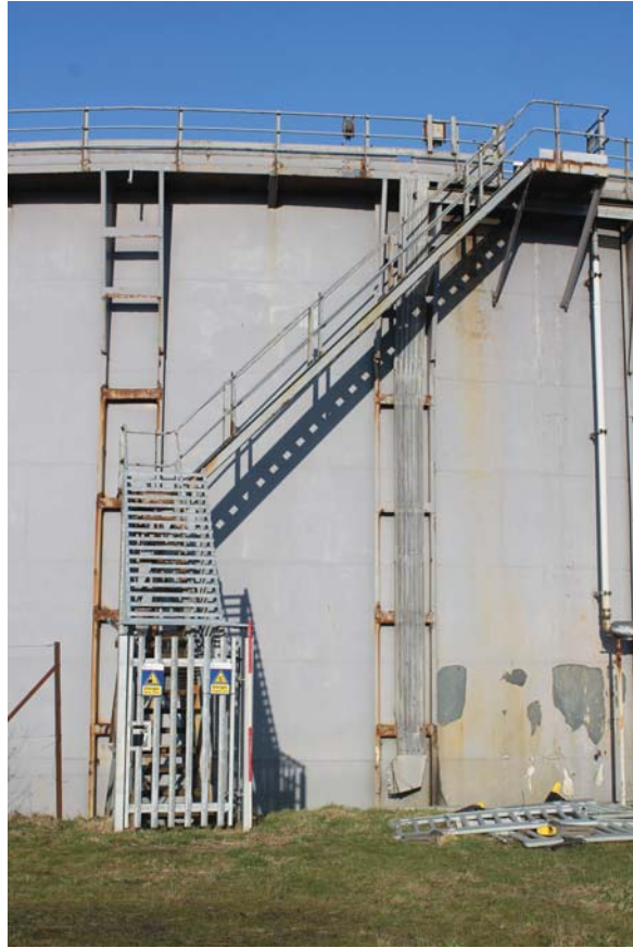
Plate 7: Weir Road, Newtown-on-Ayr, general view of stair on the south side of the gasholder from the south-east
