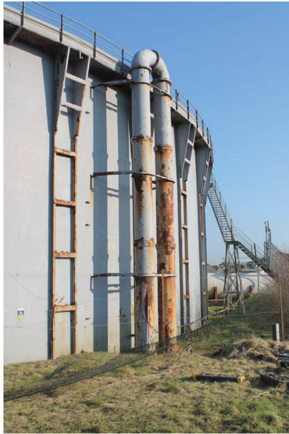
Plate 11: Weir Road, Newtown-on-Ayr, general view of pipes on the SSW side of the gasholder from the NWW
