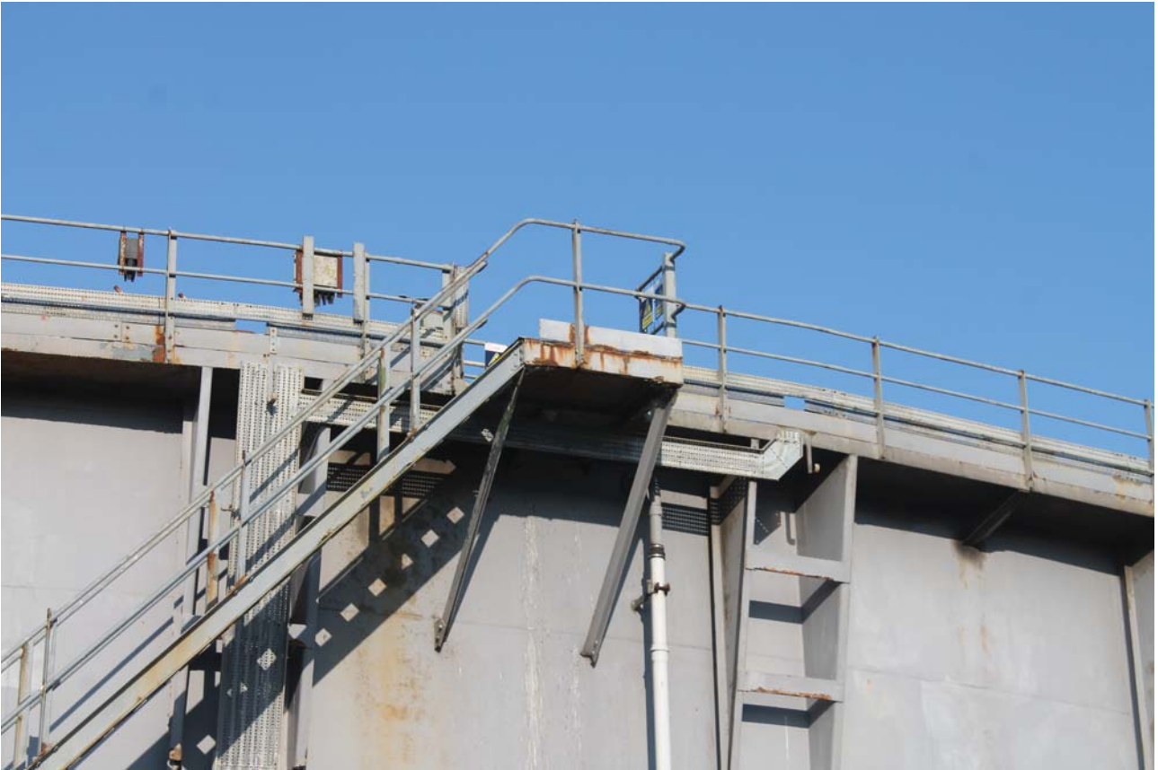
Plate 9: Weir Road, Newtown-on-Ayr, detail of the top of the stair from the south
