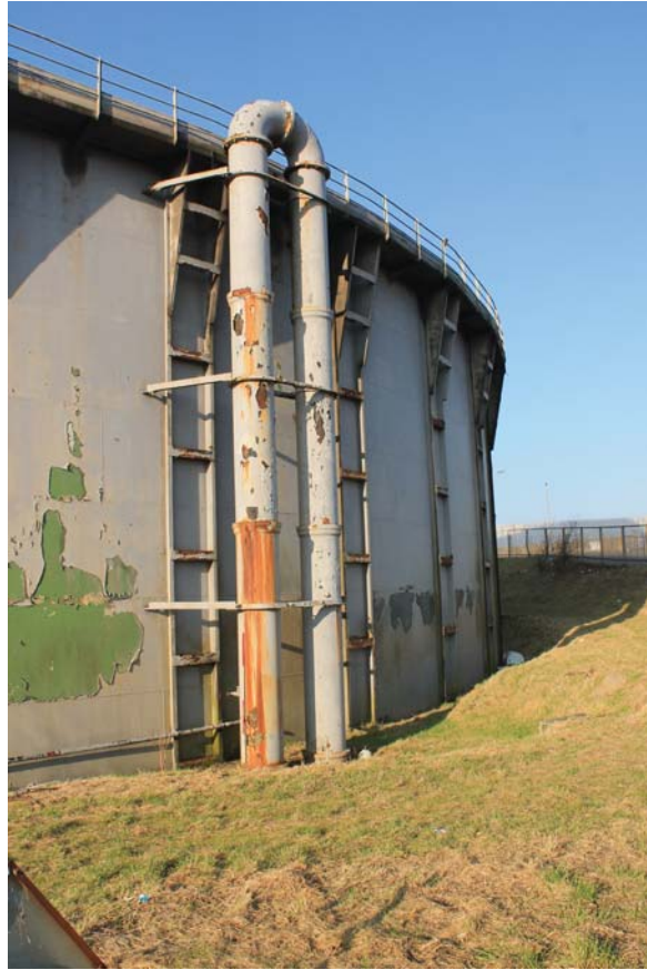
Plate 13: Weir Road, Newtown-on-Ayr, general view of the pipes on the east side of the gasholder from the south-east
