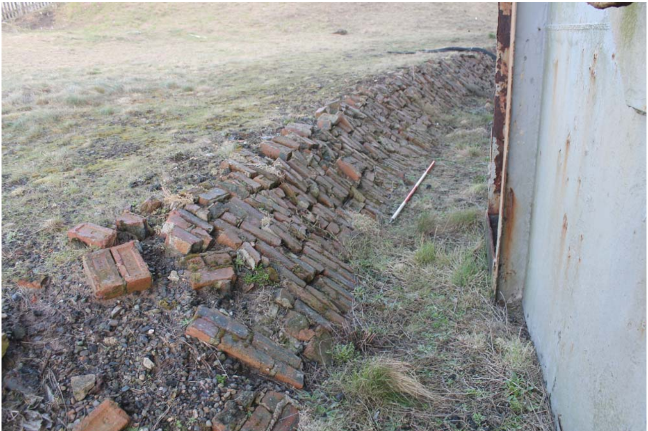
Plate 18: Weir Road, Newtown-on-Ayr, general view of brick paving to the small embankment on the north-west side, from the south-west
