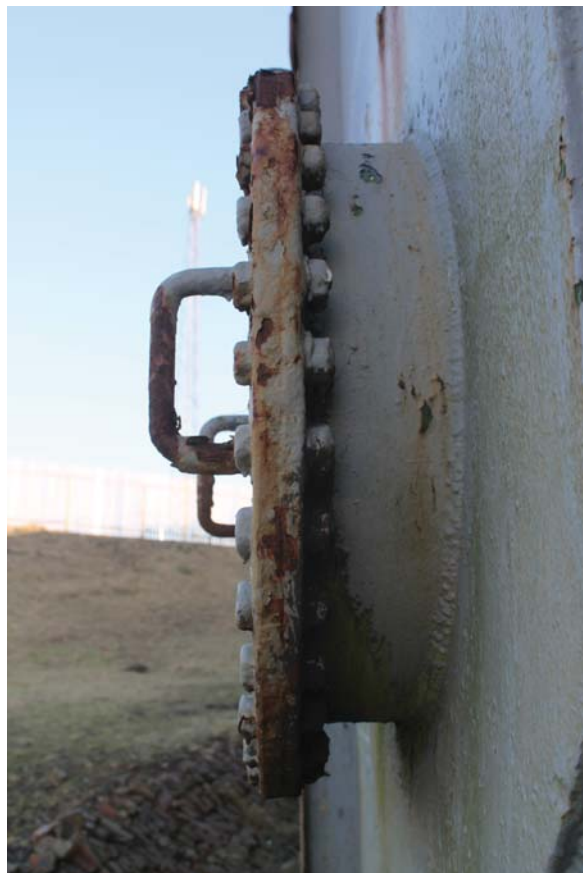
Plate 16: Weir Road, Newtown-on-Ayr, detail of the side of the inlet pipe on the north-west side of the gasholder, from the south-west
