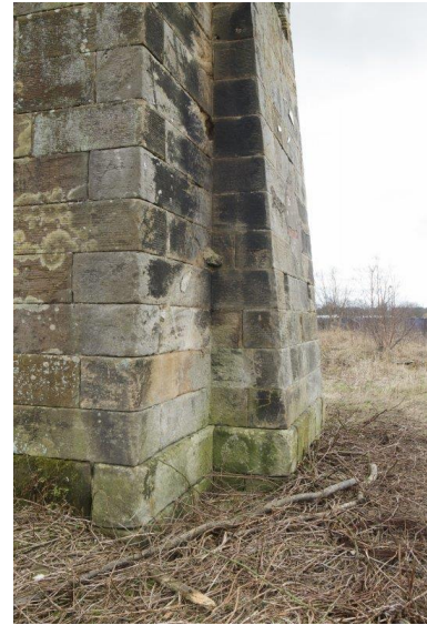
Above: View of base of west gable or 'bob wall'. The buttress would have strengthened the wall as it bore the weight of the beam of the engine where it pivoted. [DP232009, HES]
