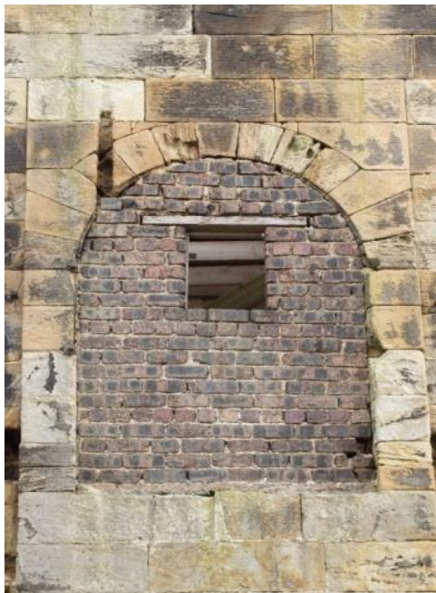
Left: View of the west or 'bob wall' opening through which the western half of the engine beam would have protruded (at Second Level). Note the remnants of handrail fixings. The groove, top left, may have something to do with bracing for the external maintenance walkway/ beam gantry (now gone). [DP232019, HES]
