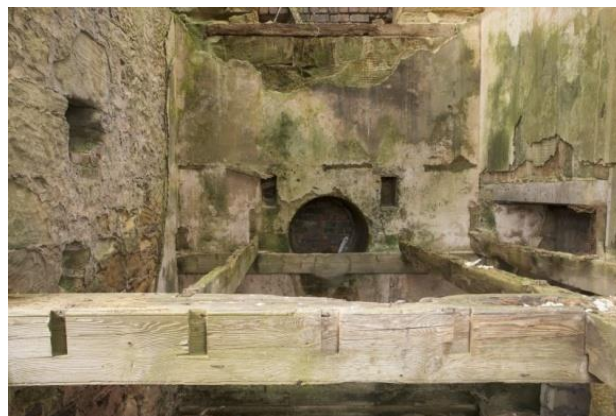
Above: View of interior, west elevation: Ground/First level. The beam in the foreground may be original and could have been part of the pumping engine [DP231996, HES]
