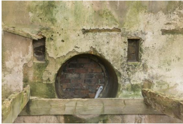
Above: View of interior, west elevation: Ground/First Level. Detail of socket holes and delivery pipe from the pump riser. [DP231999, HES]
