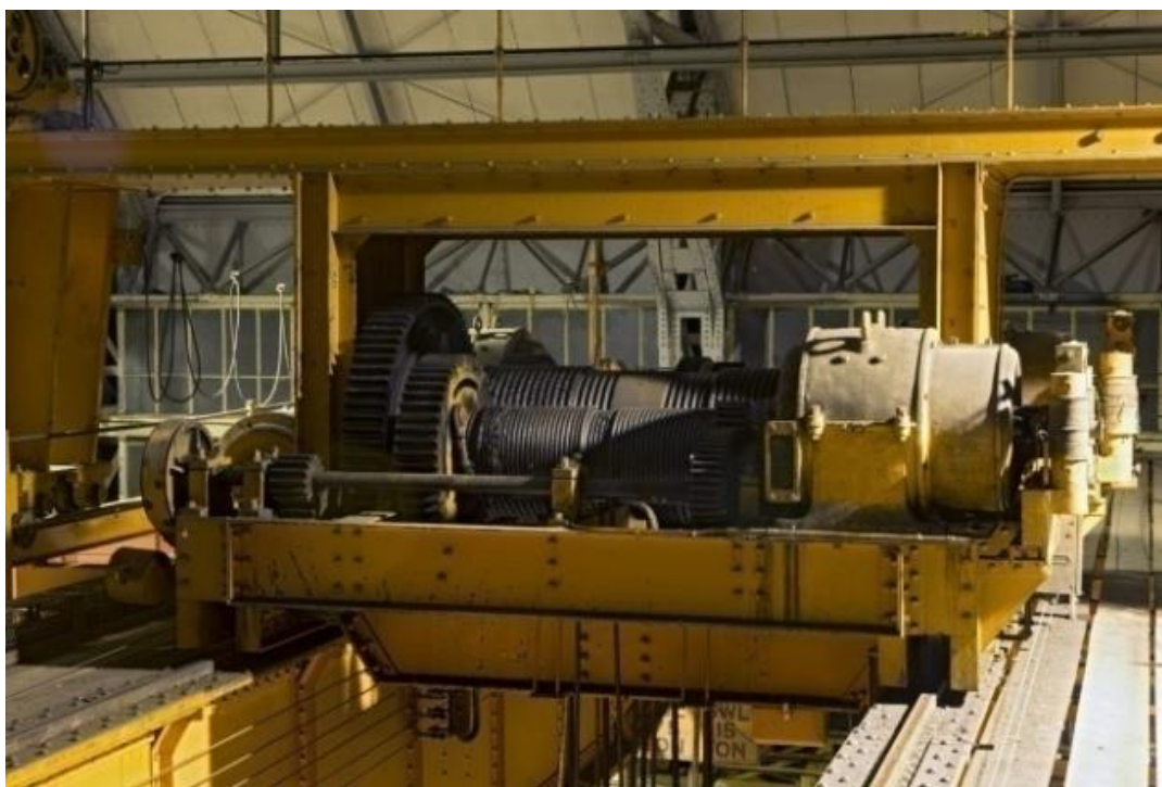
Left: Detail of south 75 Ton EOT crane, Bay C showing later structural amendments (1970s). (DP172012, RCAHMS, 2013)
