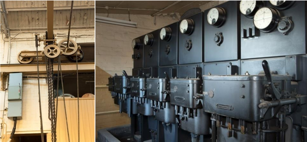
Above left: Interior of Power House; Small chain driven manual overhead travelling crane, ground floor, south end. (DP171747, RCAHMS, 2013) . Above right: Upper floor, view of transformer house switchgear (oil switches) made by Fergus Pailin Ltd Manchester - feeder units and ammeters (DP171755 , RCAHMS, 2013)
