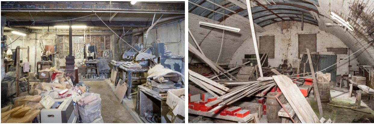
Left : interior of ground floor of Dalmore Mill from south. Diamond saw cutters line the walls. The replaced steel joist and concrete ceiling is just visible. Right: interior of Storage Shed no.1 from south. Note the collapsed wooden roof lining and the completed industrial hones below. These were stored by size.
