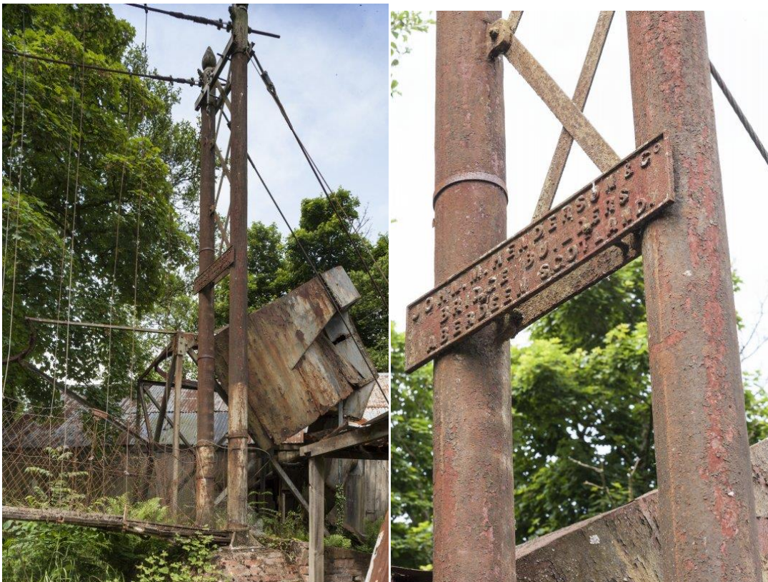
Left: View of north pillars, anchor cables (right) with the mesh protection and the deck of the bridge visible on the left (DP161956) and detail of north pillars makers plate [DP161957, 2013, RCAHMS]
