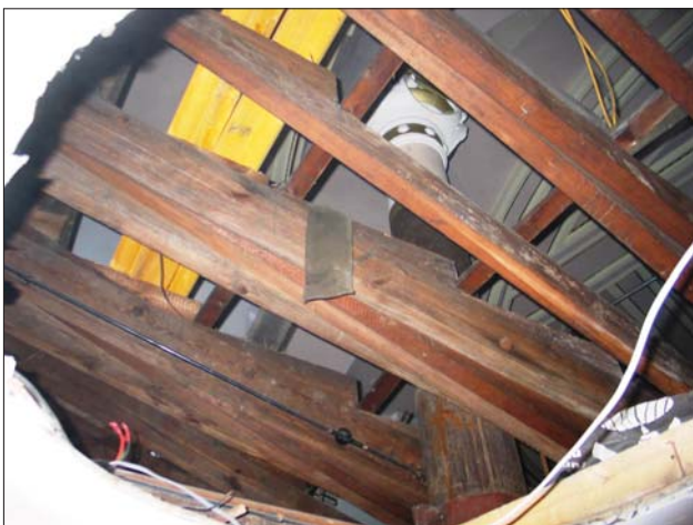
Plate 11: Detail of the timber floor beams of balcony from below. Looking towards ceiling of auditorium.
