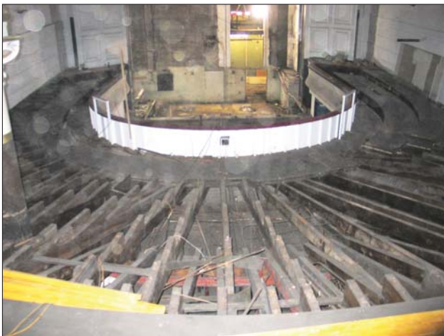
Plate 9: Timber floor beams after the removal of the early raked floor. Looking north-west.
