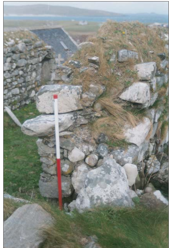
Plate 8: Building No.3, South Wall interior; collapsed masonry and internal quoins at SW corner of primary building, facing NE.
