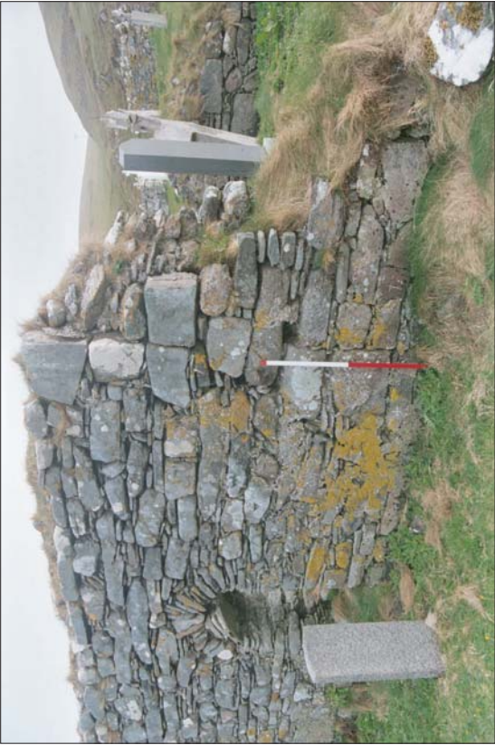
Plate 12: Building No.3, North Wall exterior; detail of butt joint between primary and secondary wall fabrics, facing SE.
