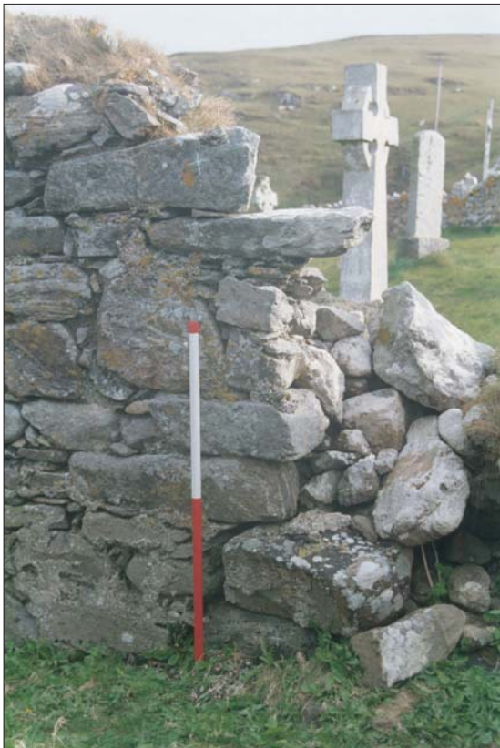
Plate 7: Building No.3, South Wall interior; collapsed masonry and internal quoins at SW corner of primary building, facing SE.
