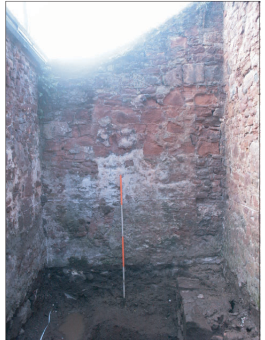
Plate 2. (right) The west wall - The clay bonded walls (20,21) scarring (22) and upper coursing are visible.
