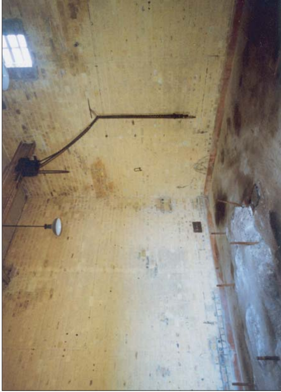
Plate 15 - The interior of the generator house (TJ)
