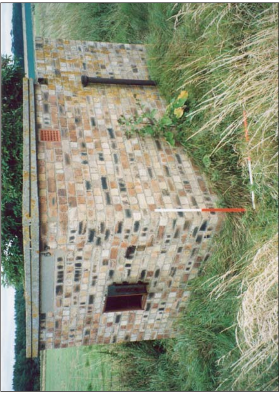
Plate 26 - The IFF cubicle from the northwest
