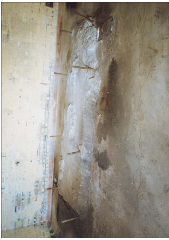
Plate 16 - The interior of the generator house (TJ)
