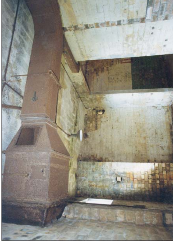
Plate 11 - Part of the air filtration system (TJ)
