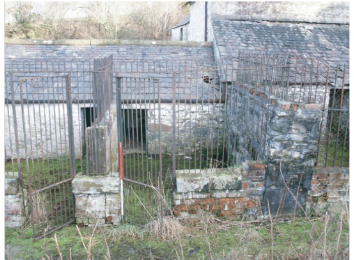
Plate 16 : Buildings C and D. The kennels, west exterior elevations. Note the contrast between the two types of railings and the different brick types between the two phases of construction.
