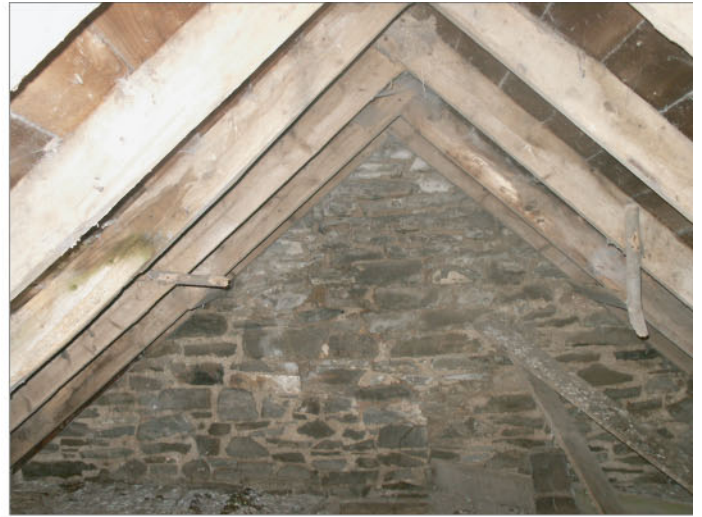
Plate 14 : Building B, Room 4. East interior elevation. The loft space appears never to have been lime washed. The roof trusses and sarking are original.
