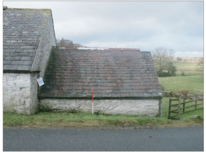
Plate 2 : Building B loft, Room 4. South exterior elevation. Blocking for chute is central and partly obscured by modern ground surface. Compare colour of tiles with those of Building A.
