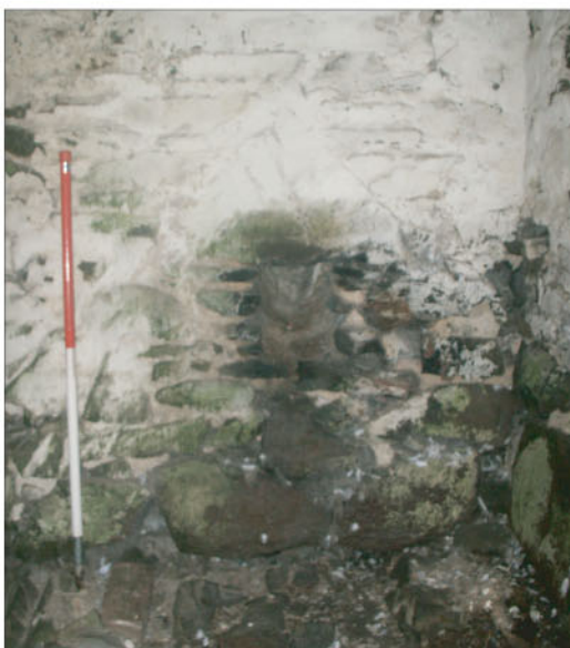
Plate 11 : Building B, Room 3. East interior elevation. The chimney flue. Note triangular arch and narrow opening.
