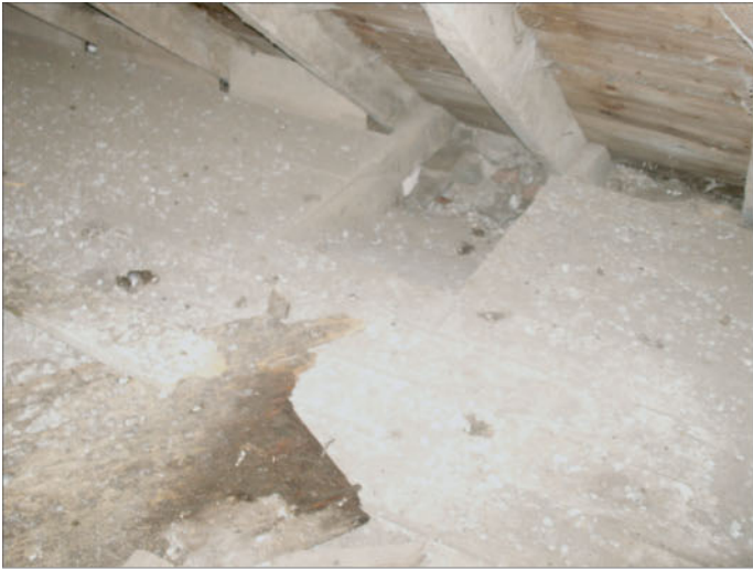
Plate 13 : Building B loft, Room 4. South interior elevation. Detail of chute. Floorboards directly overlie tie-beam of trusses. Note angled plank between floor and sarking in eaves space.
