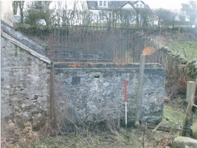
Plate 15 : Building D. North exterior elevation. The loop-headed railings are set into bricks over a concrete coping.
