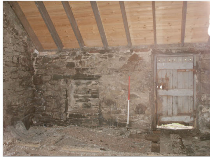
Plate 8 : Building A, Room 1. South interior elevation showing doorway and blocked window. The original floorboards are rotten and in a dangerous state. The roof construction is a modern replacement.
