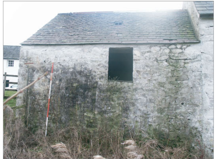
Plate 4 : Building B Room 3. North exterior elevation showing window. Kelton Mill is to the rear.
