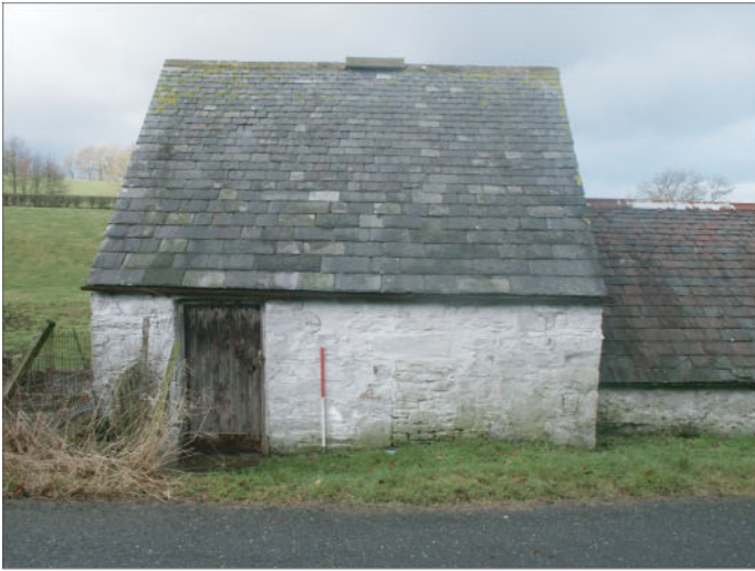
Plate 1 : Building A - Room 2. South exterior elevation showing doorway and blocked window. The building has been recently re-roofed. The modern ground surface may be higher than contemporary with the building.
