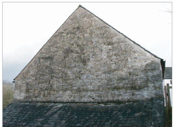
Plate 6 : Building A. West exterior elevation, gable (Room 2) above Building C the earlier kennels. The single-pitch roof is part bonded with the wall and sealed with flashing.
