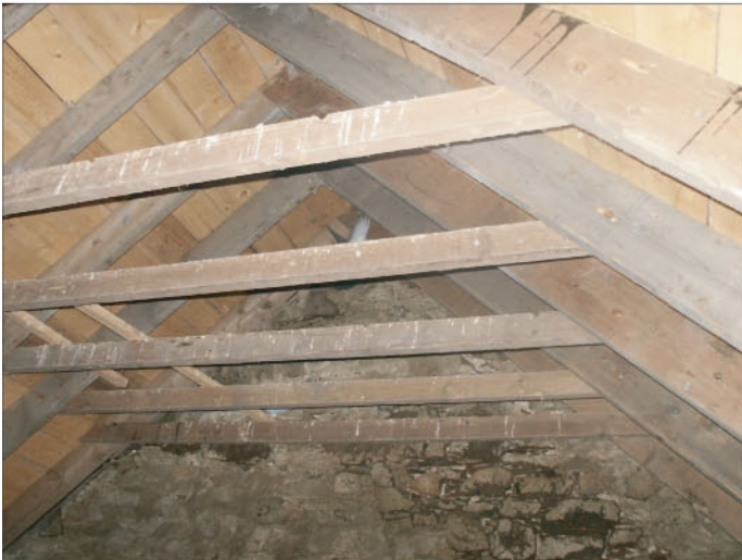
Plate 9 : Building A Room 2. View of modern roof trusses and sarking showing bolted together collar beams and rafters.
