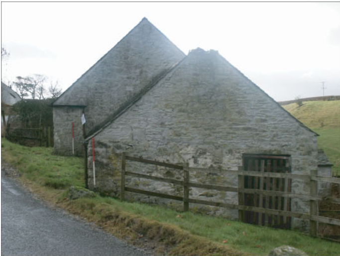
Plate 3 : Buildings A and B. East exterior elevation shows doorway and level courses in gable masonry. The chimney stack is missing and the flue has been sealed.
