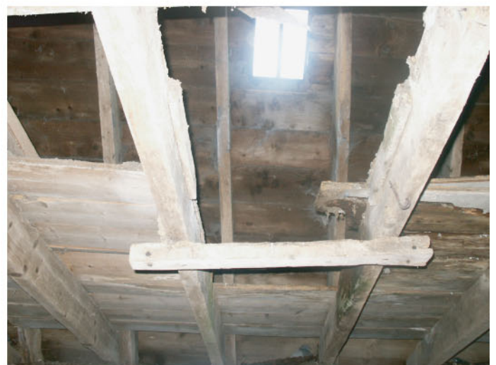
Plate 12 : Building B, Room 3. Location of trap access to loft space, Room 4. Note sawn floorboards and batten to support ladder.
