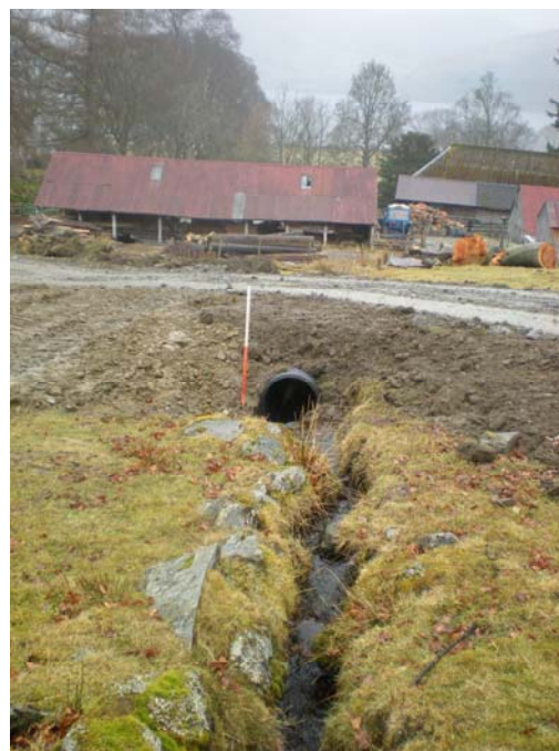
Site 19 drain showing new pipe under built up upgraded track and farm buildings Site 23 in the background.
