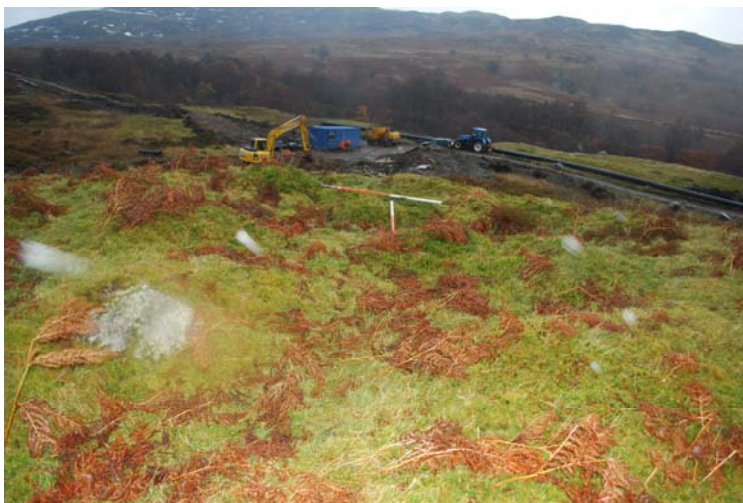
Shieling hut Site 2.63, view to the W towards route to Intake 5 and working compound.
