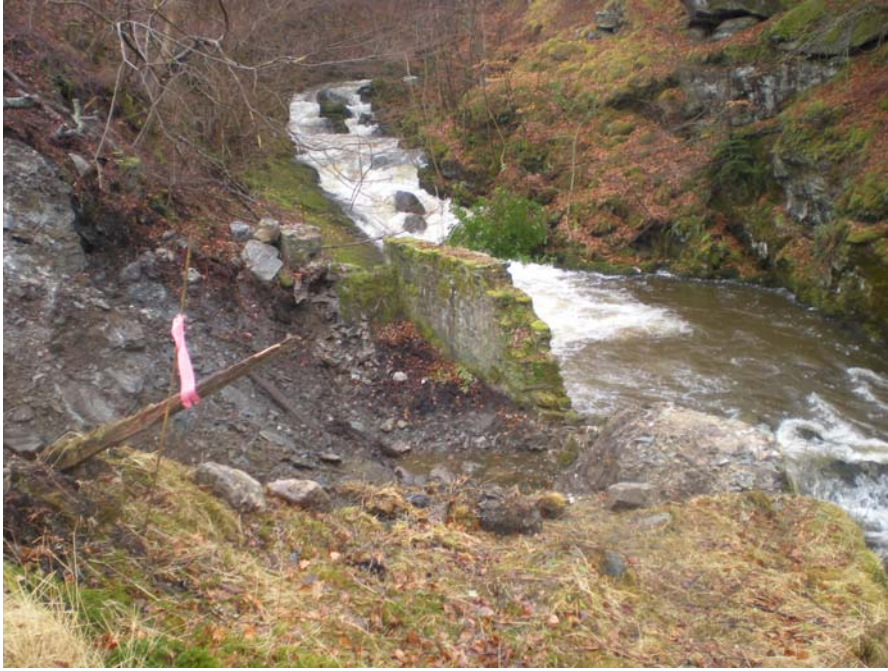
View of the saw mill Site 22 following demolition, note the S and W walls of the wheel pit (Elements 5 and 7) have been retained.
