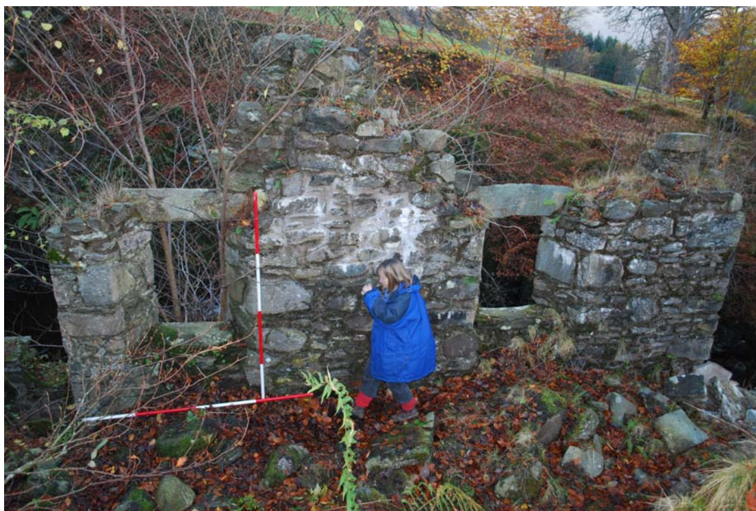
The interior elevation of the W wall of the mill building, Element 10 and Jennifer Robertson. Note the collapsed stones in the interior. View to the W.
