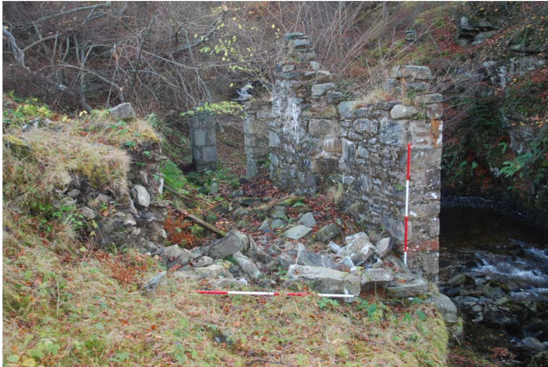
View to the S of the interior of the saw mill building showing the interior of the W wall Element 10 and aperture to the wheel pit. On the left side of the photograph the collapsed E wall and exterior platform are visible.
