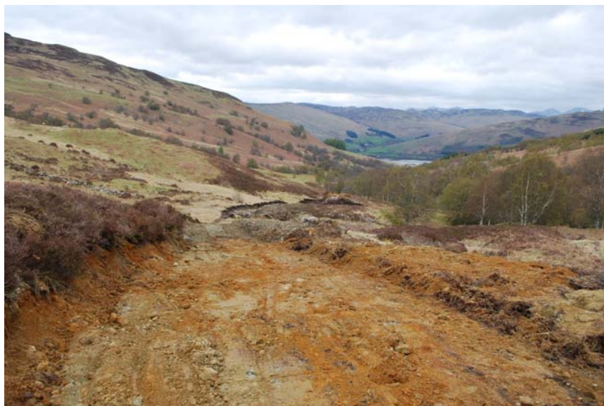
General view to the NW over the pipe route to Intake 6B.
