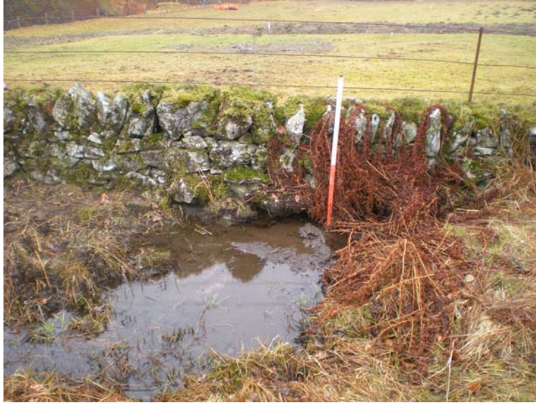
Culvert 18A, badly silted up, on the south side of Wall 18, View to NW.
