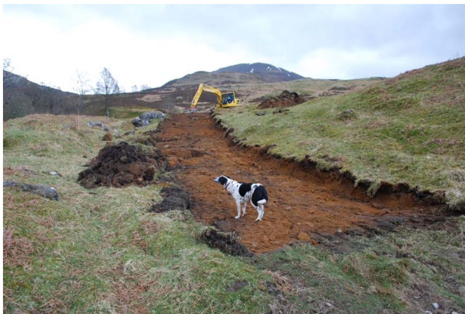
Excavation of existing track Site 4 to upgrade it and install pipe and knoll that was cut back on the right of the picture. View to the S, machine is at the turn to the W to Intake 5. Individual spoil heaps utilised to avoid dumping on shieling sites.
