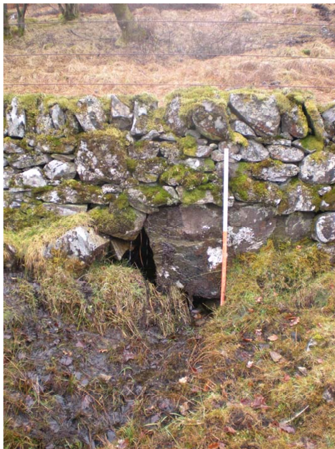
Culvert 18A, on the N side of Wall Site 18, start of drain Site 19. View to SSE.
