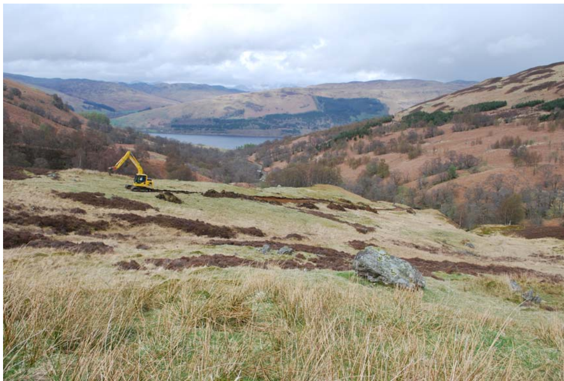
View over excavations of pipe route to Intake 5, view to the N from Site 2.55.
