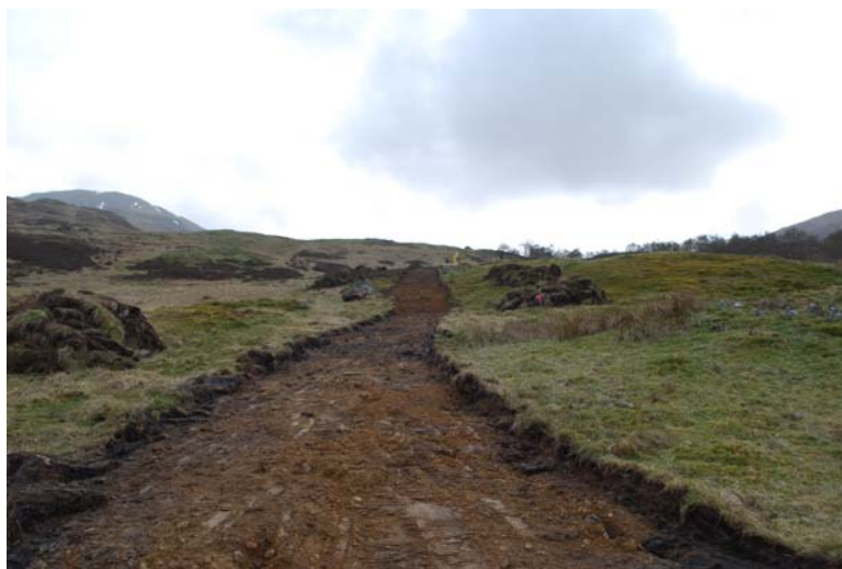
View to SW along pipe route to Intake 5 as excavated from the junction with existing track Site 4.
