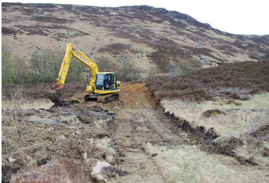
General view to the E over the pipe route to Intake 6B.
