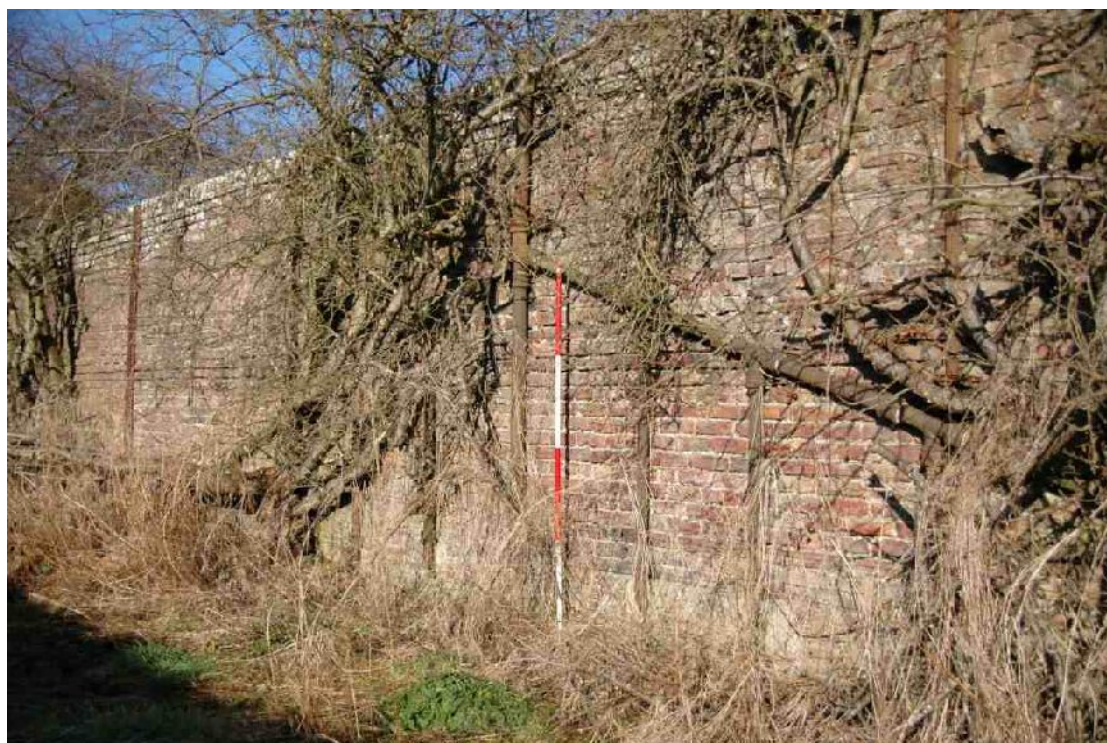
Illus 99 Pipe-work of heated peach wall
