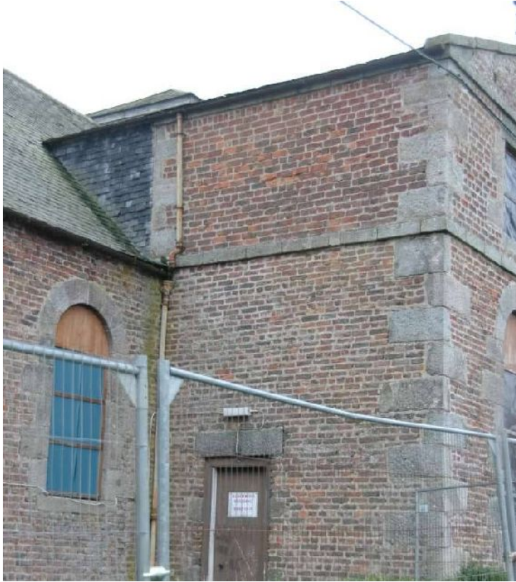
Illus 30 N angle of projecting central block of chapel showing difference in brickwork above the string course
