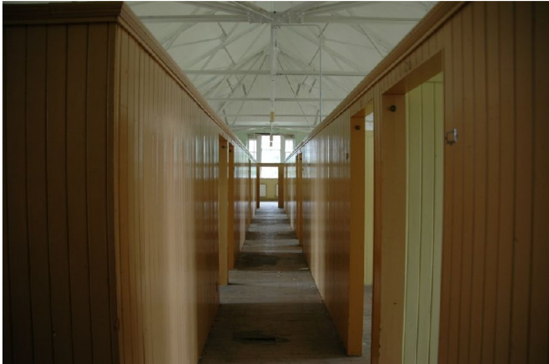
Illus 84 Individual cubicles for older boys in the 2 nd floor of the 1906 extension. Note the cast iron roof.
