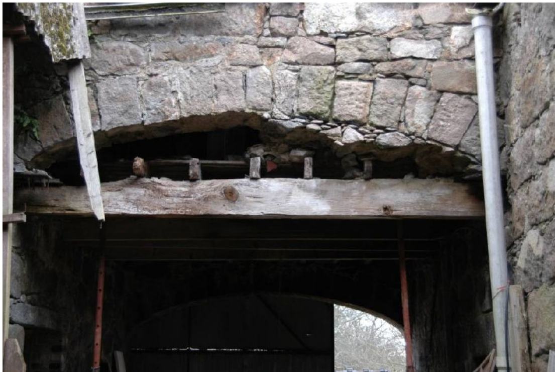
Illus 117 S (Inside) of archway over road into courtyard. Building 10 RHS, Building 13 LHS. Attic continued across above arch.
