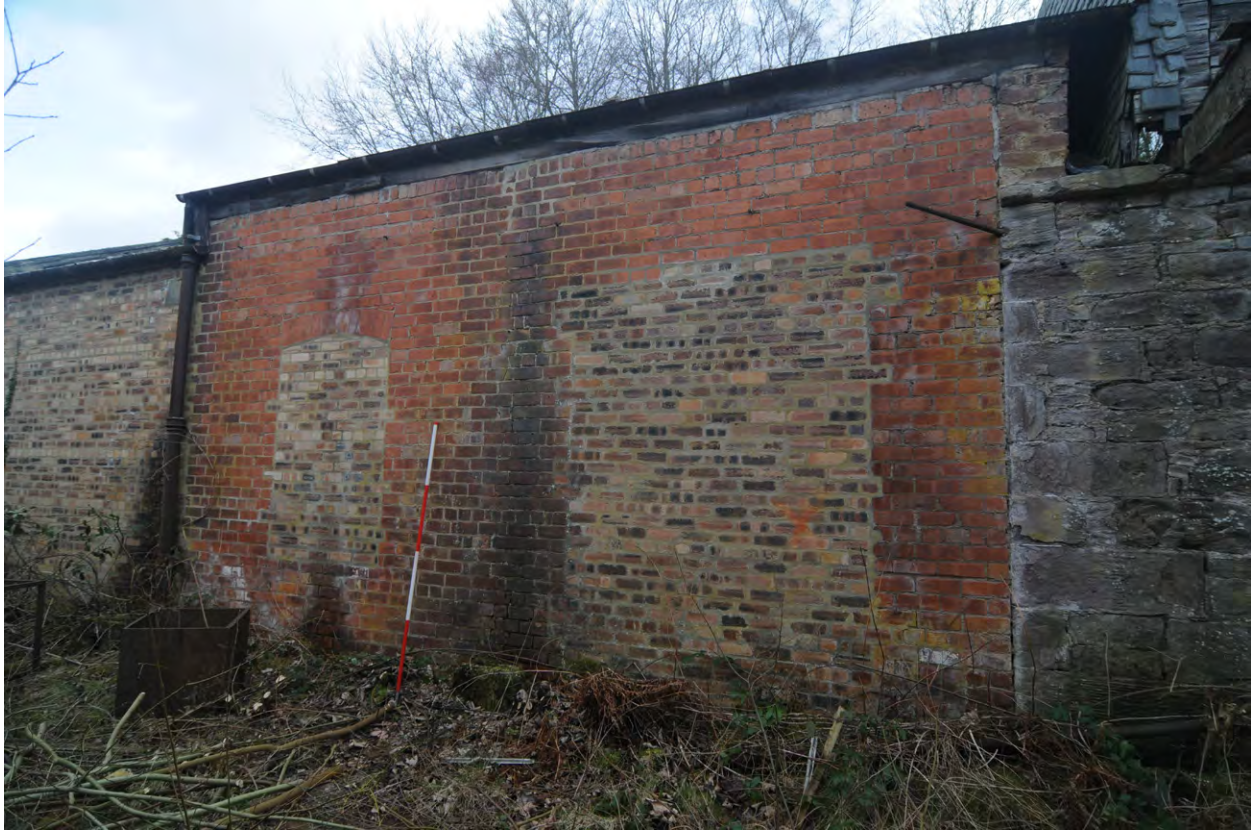
Fig 17: Phase 4 external west-facing elevation, Unit 3, showing window (038) and doorway (039) both blocked in Phase 5
