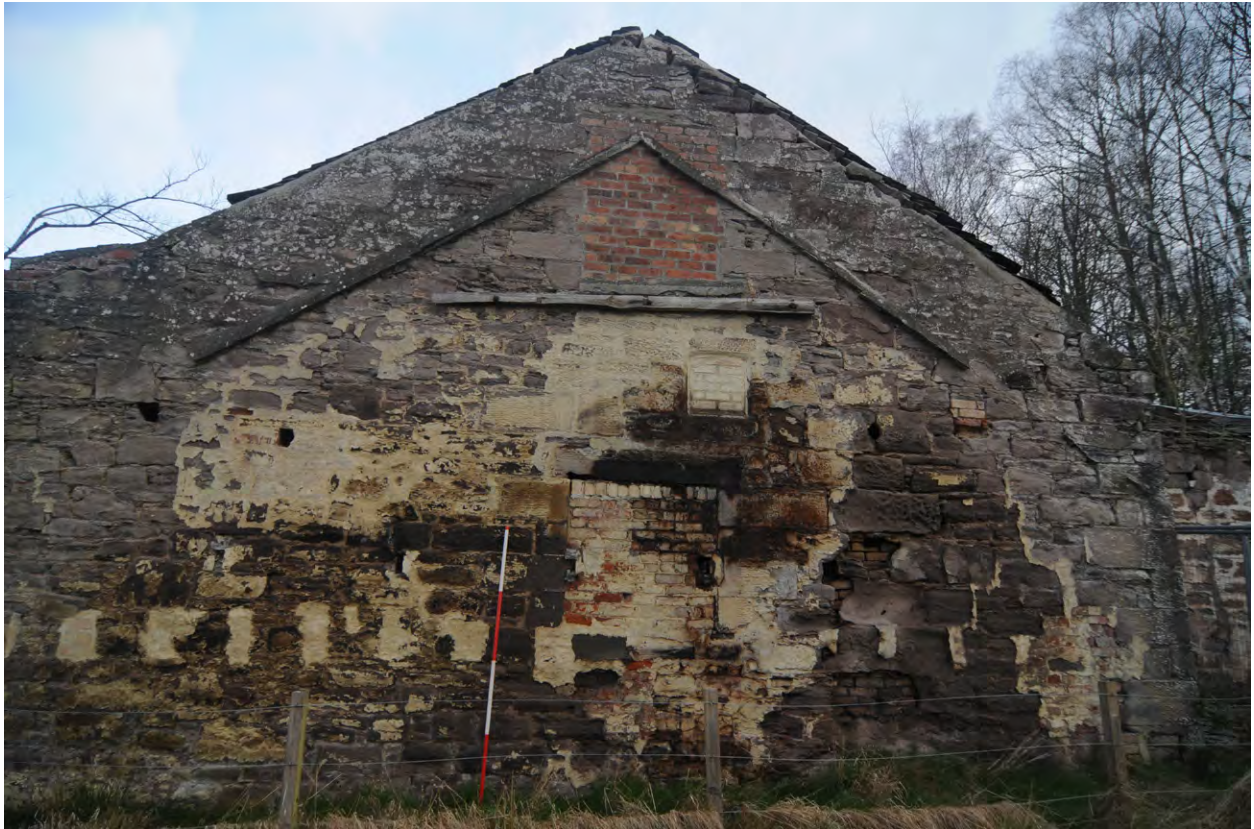
Fig 10: Phase 2 remains of raggle line of missing building and blocked windows (003) and (007)
