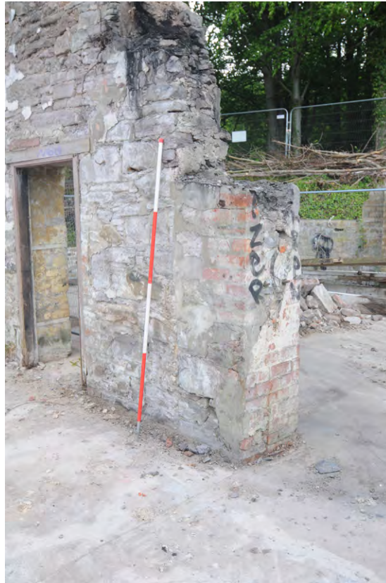
Fig 18: Phase 4 Unit 2/3, remains of brick support column (053) for roof support I beam
