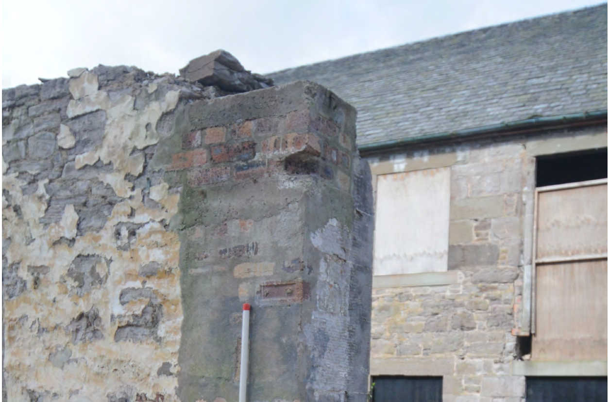
Fig 19: Phase 4 Unit 2/3, remains of brick support column (054) for roof support I beam
