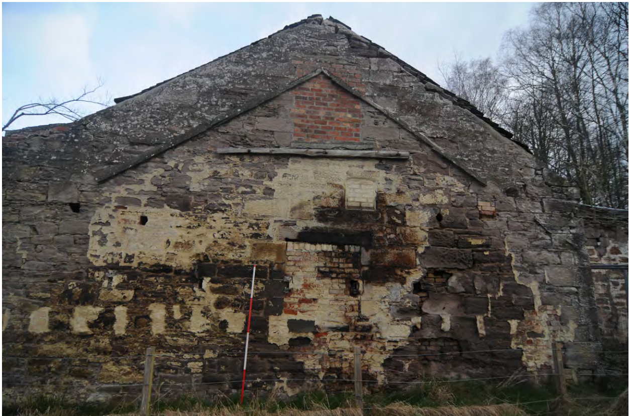
Fig 10: Phase 2 remains of raggle line of missing building and blocked windows (003) and (007)
