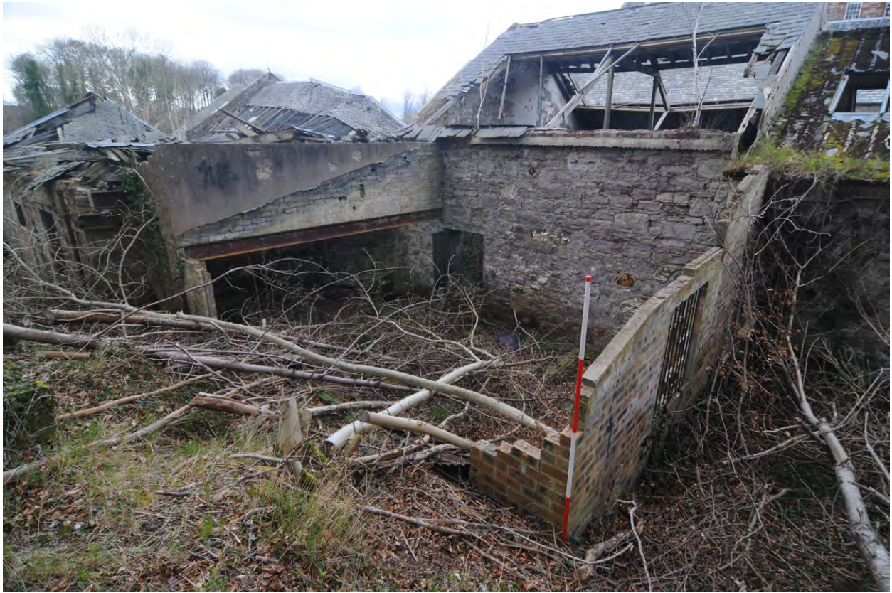
Fig 27: Phase 7 Unit 5, external east and north-facing elevations showing damage caused by vandalism and raggle line for sloping corrugated roof
