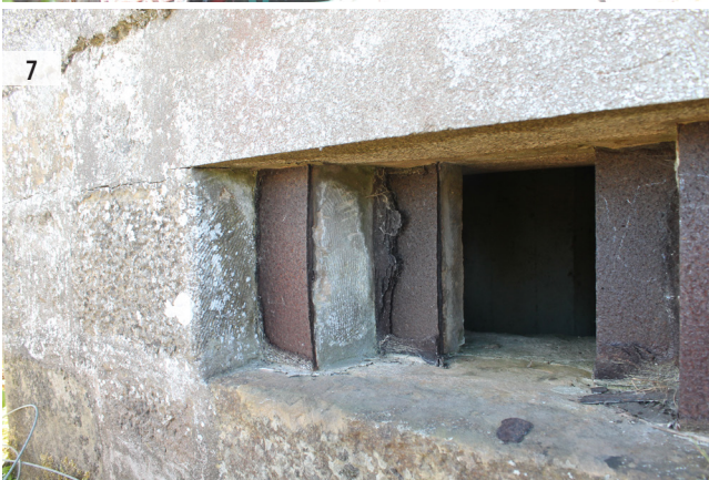
ILLUS 3 General view of the pillbox facing west ILLUS 4 Detailed view of the underside of the concrete roof ILLUS 5 Detail of the entrance blast wall facing north-west ILLUS 6 Detail of the loophole on the north facing wall ILLUS 7 Detail of the stepped opening of the loophole
