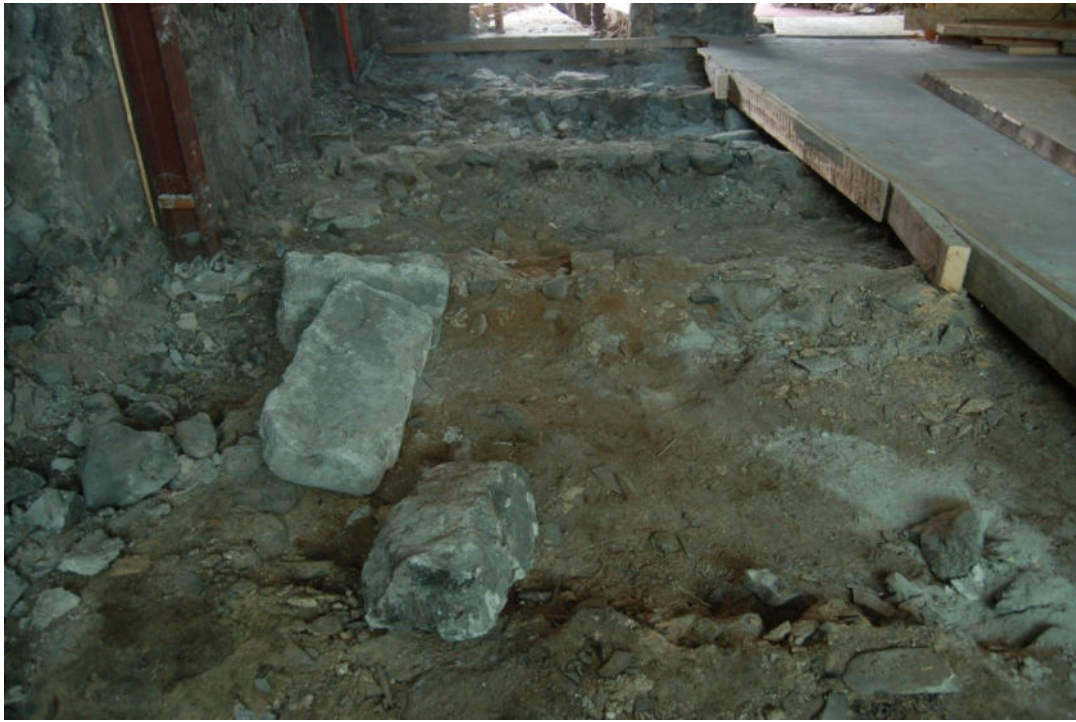
Illus 5 Sleeper walls exposed by removal of floorboards within the retail space fronting onto High Street; facing S.
