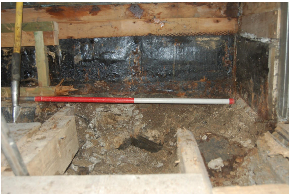
Illus 15 Working shot of Trench 3 showing the granite foundation of the N wall supporting an I-beam and window above; facing N.
