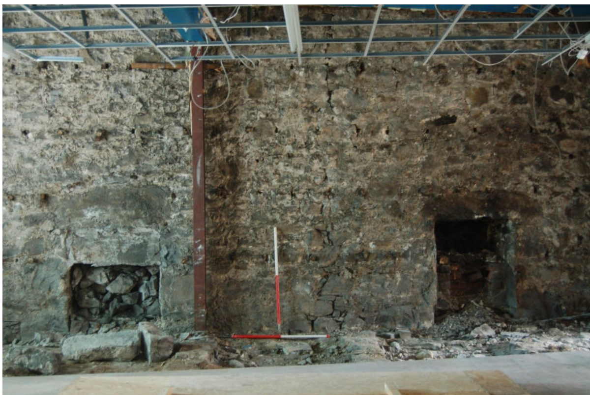
Illus 2 WNW facing elevation within the front existing retail space; facing ESE.
