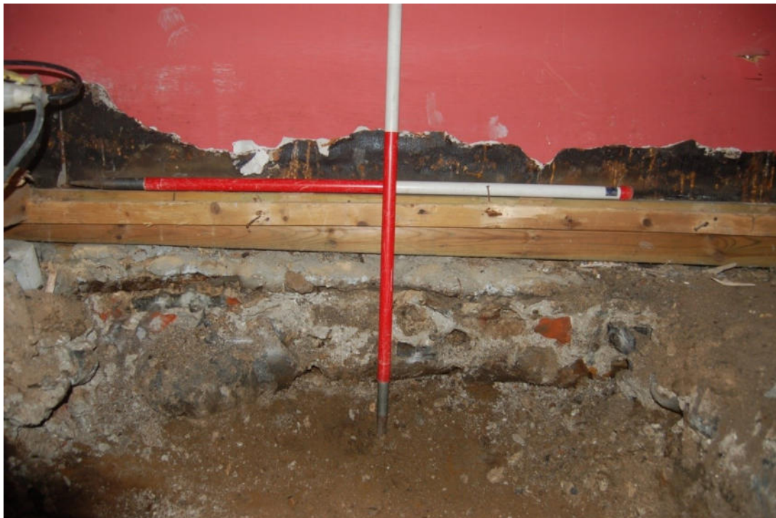
Illus 13 Foundation of the N wall of the structure fronting onto the High Street, beneath the frame of a modern floor-to-ceiling window; facing N.
