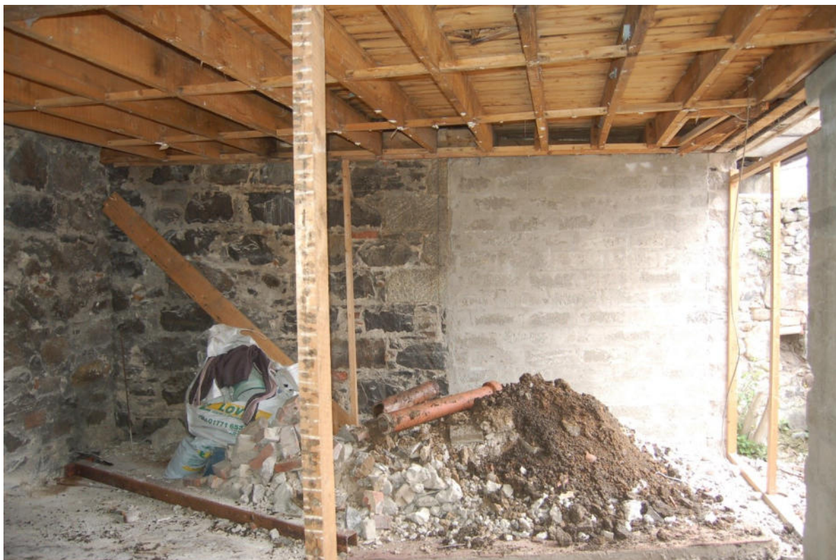
Illus 7 Working shot showing the modern cement block extension built onto the earlier granite structure of the ESE wall; facing ESE.
