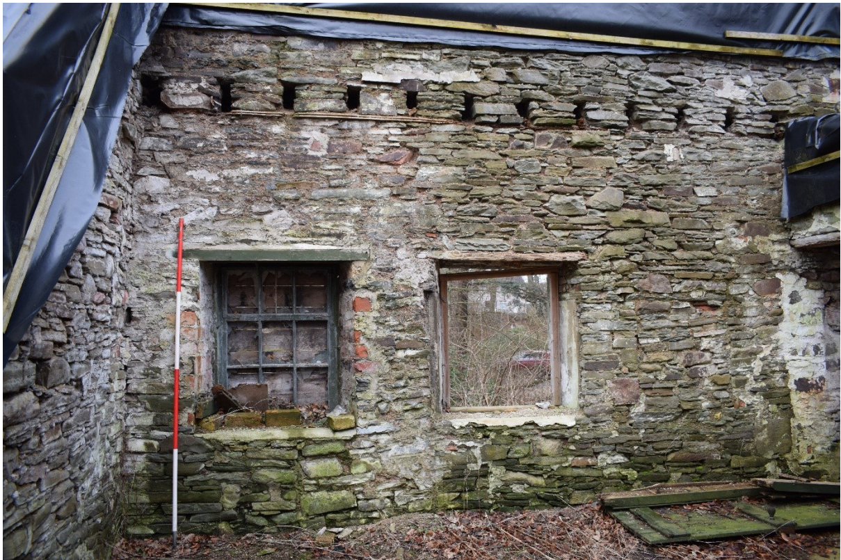
Illus 14 Interior SSE wall Room 3 W6 (left) W5 (right) with beam slots above; facing SSE
