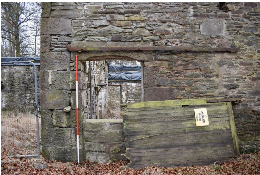
Illus 28 NNW wall Room 2 D2 with arched sandstone lintel and lower half blocked; facing SSE
