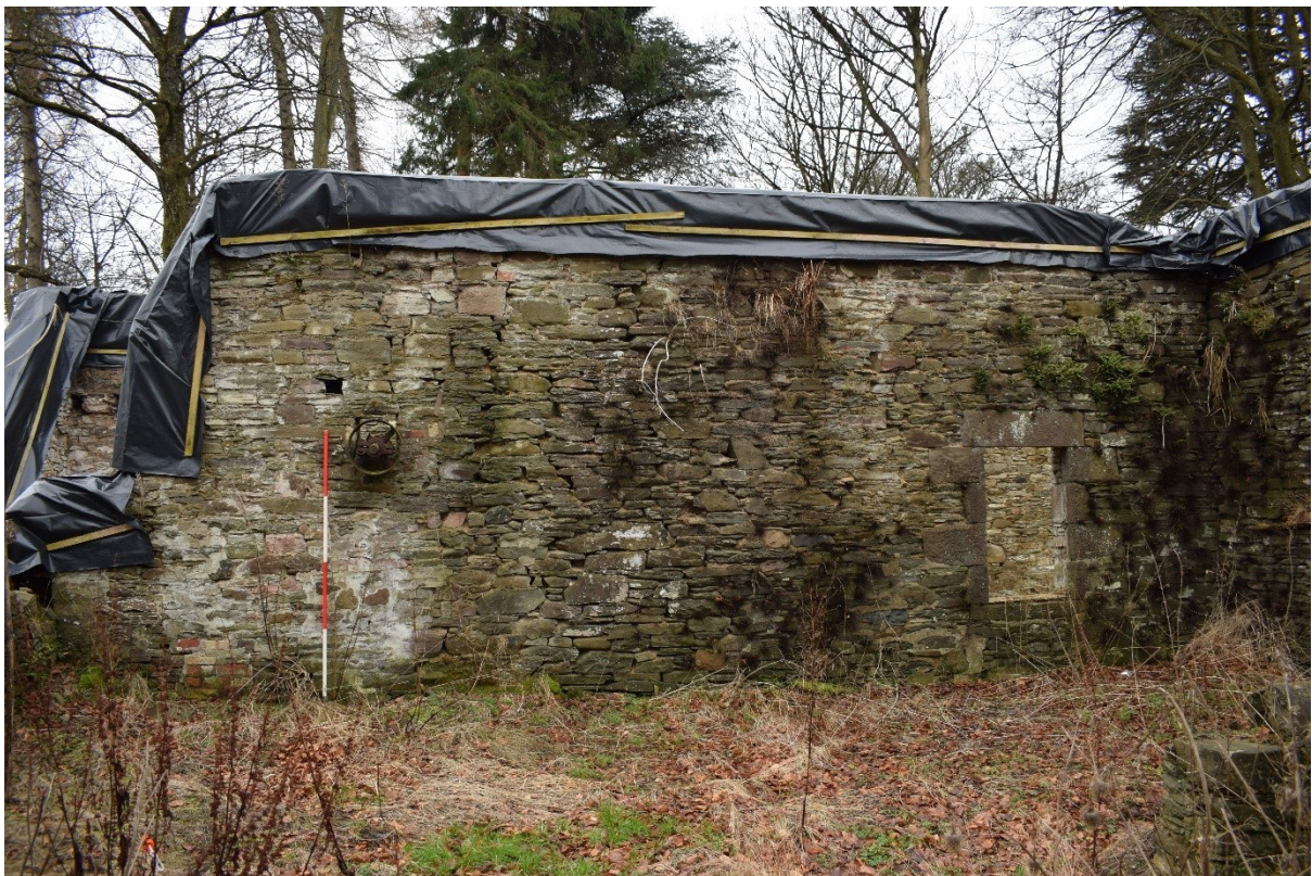
Illus 20 NNW face of Room 1/Room3 wall with vent F16 (top left), F6 and W7 (right); facing SSE
