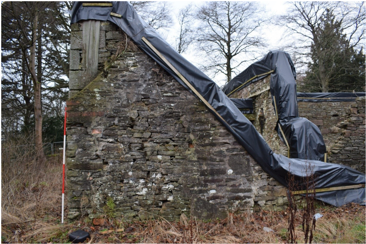
Illus 11 ENE wall Room 3 in poor condition, partially demolished, possible infill in Phase 2; facing WSW
