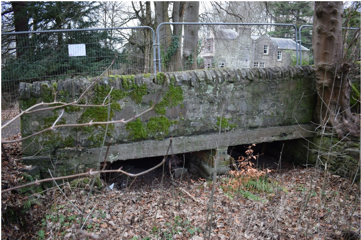
Illus 18 Detail of bridge F19 divided into lade to wheel (F18; right) and overflow lade (F21; left); facing WNW
