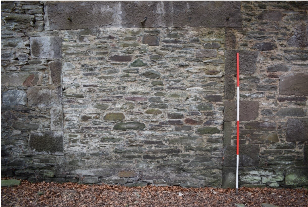
Illus 27 D1 blocked cart door WSW wall Room 1; facing ENE
