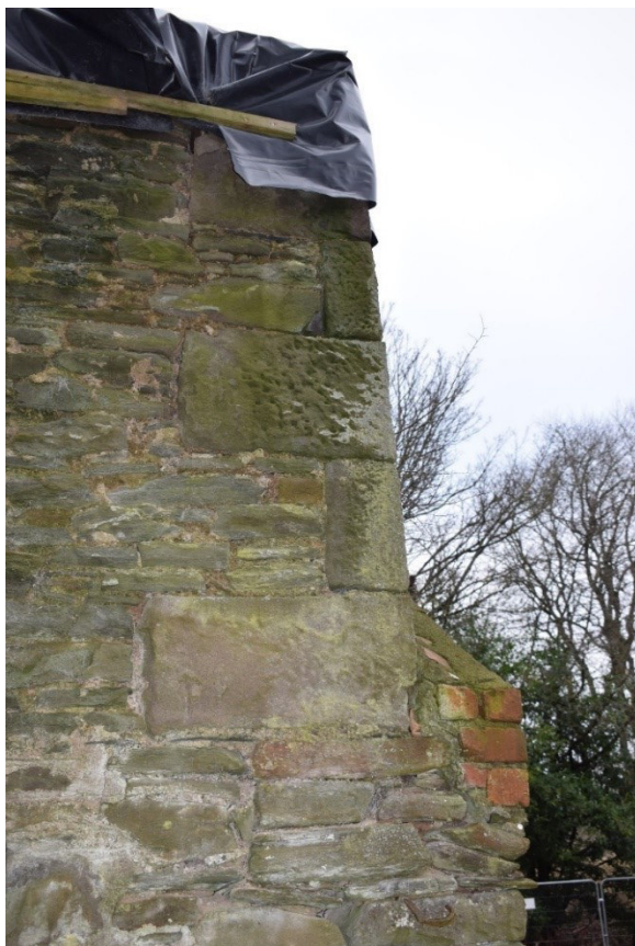
Illus 8 Phase 2 quoins SE corner above Phase 1 grey sandstone rubble wall; facing NNW
