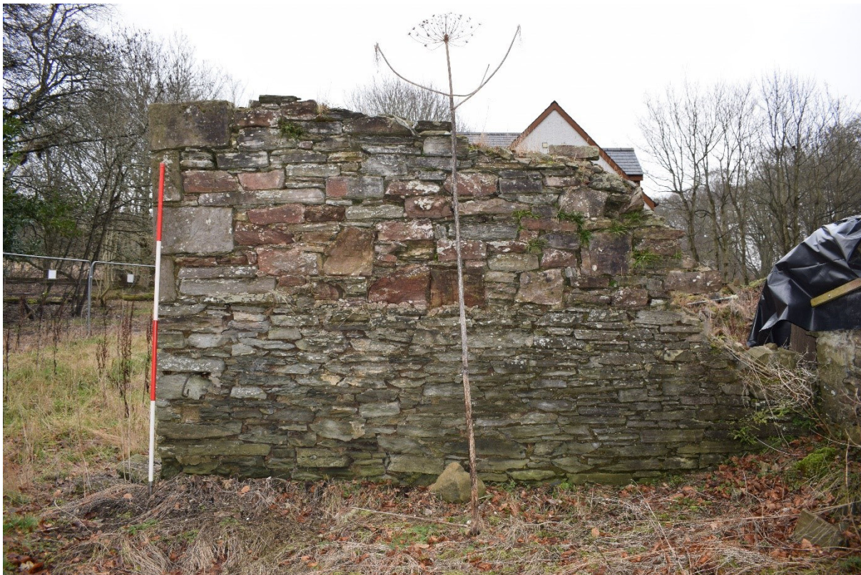
Illus 10 Wall F27 showing lower (earlier) half grey sandstone and upper half with quoins and red sandstone rubble; facing ENE
