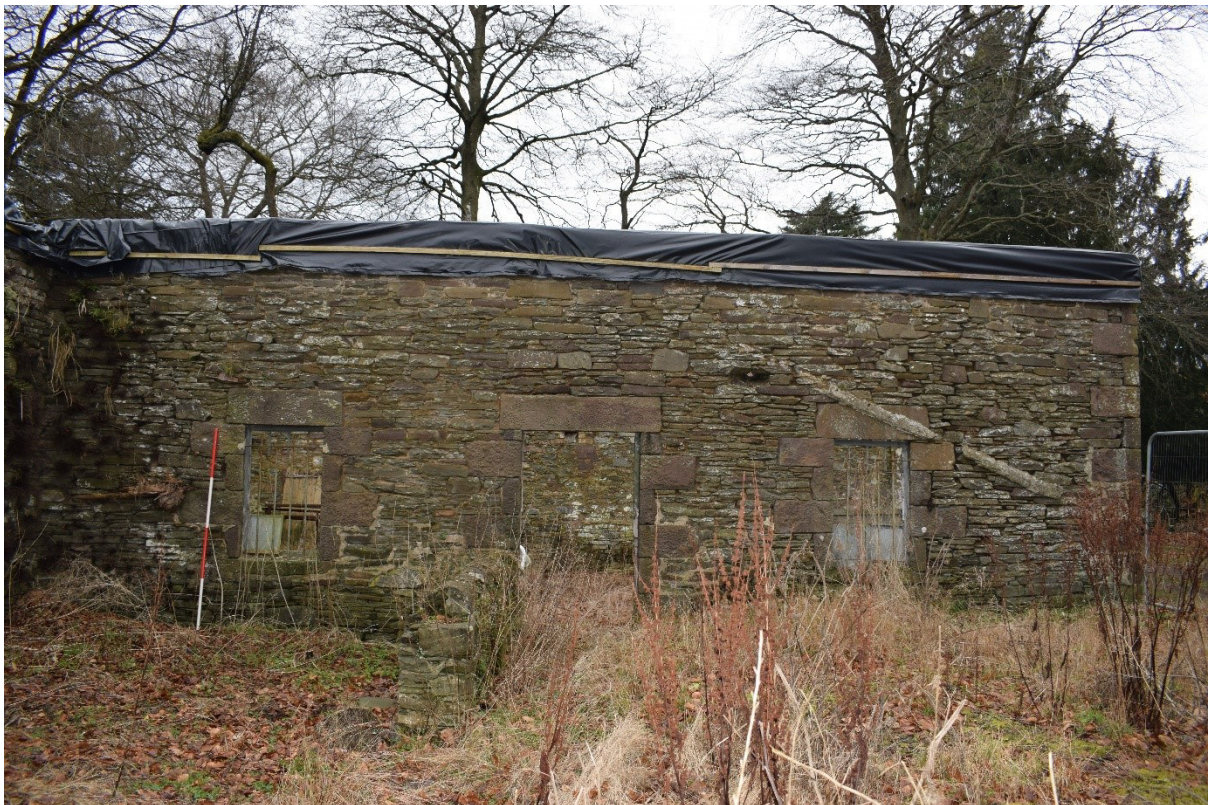
Illus 24 ENE wall Room 2 former stables with W8 (left), D6 (centre) W9 (right with roof scar F22 above; facing WSW
