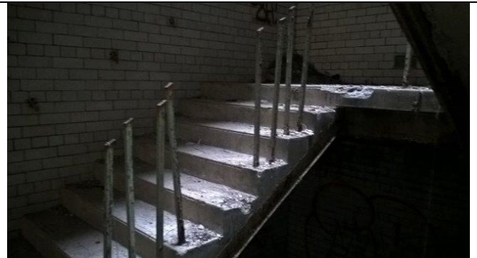
No edge protection on many flights of stairs
