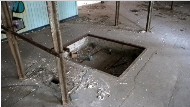
Potential trip hazard on slab
