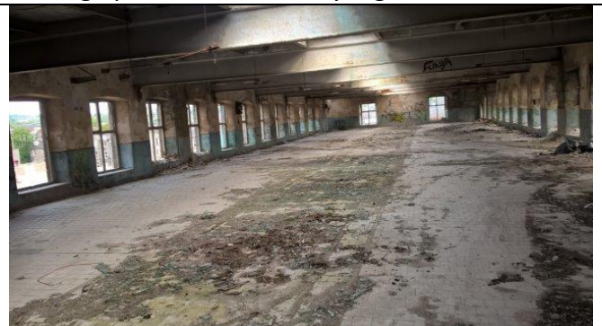
Where window frames are missing potential for fall from height.
