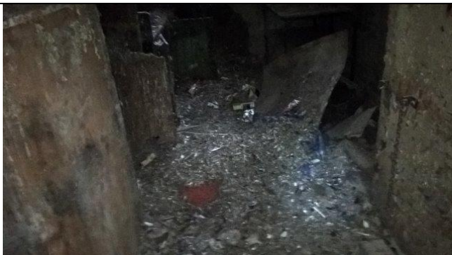
Condition of burnt out areas on ground floor
