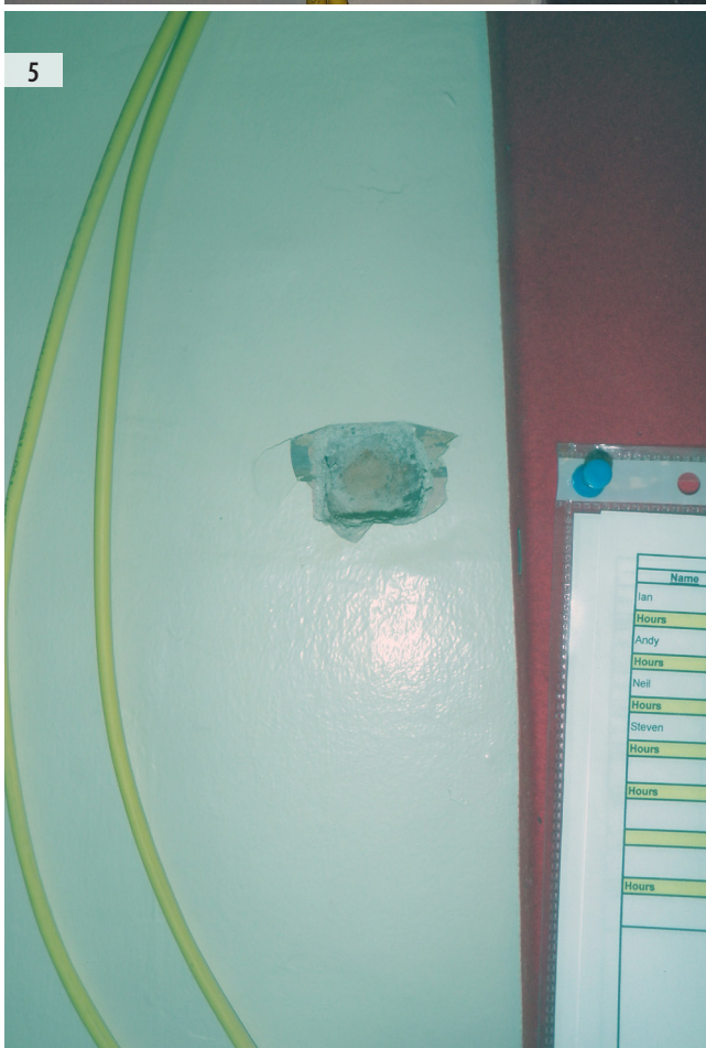
ILLUS 3 Additional damage to the plaster after removal of the rawl plug from the bottom hole on the south-west wall ILLUS 4 Exploratory hole into plaster around Hole 11 showing area of damage ILLUS 5 Exploratory hole into plaster around Hole 12
