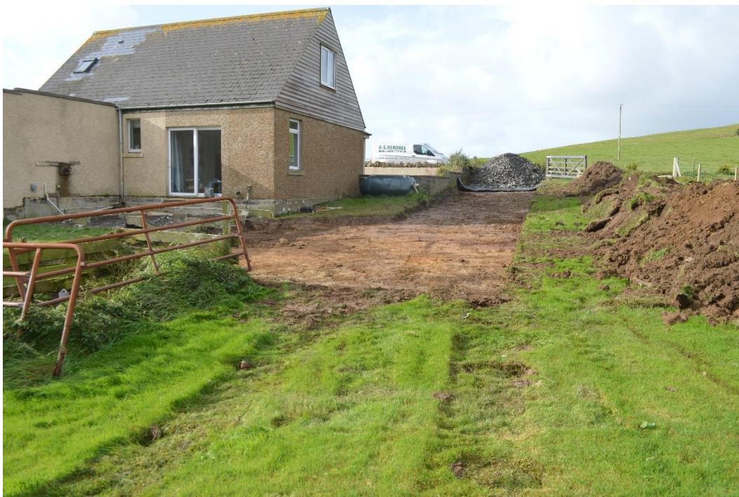
Plate 2: General view, looking west, of the temporary access road, working area and former patio following completion of the topsoil strip.
