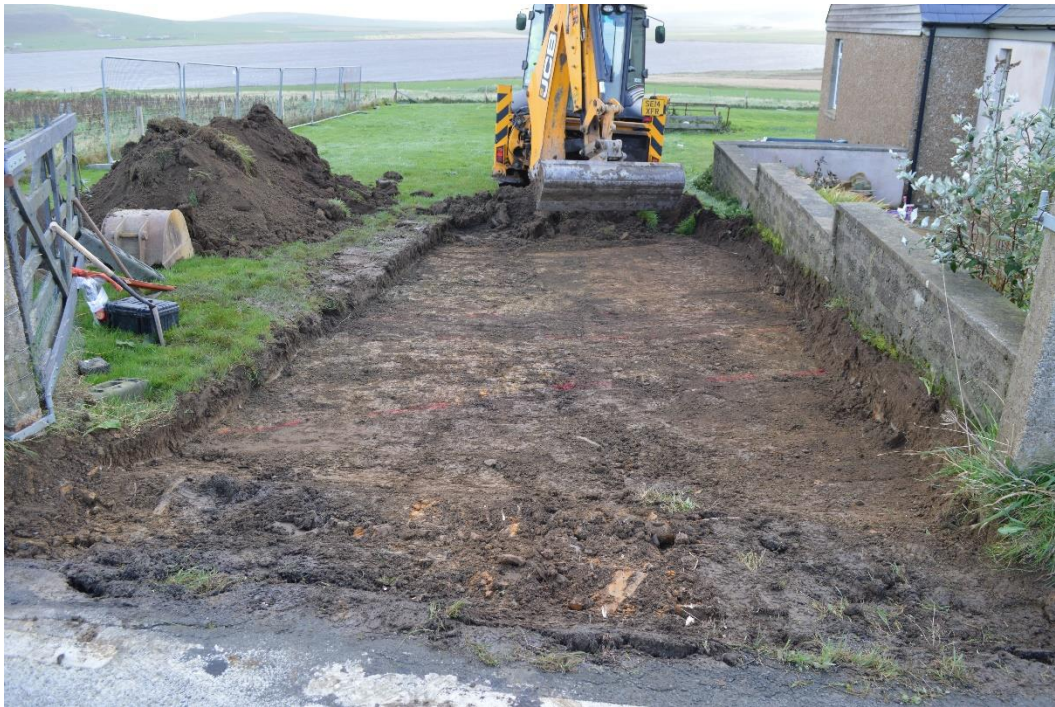
Plate 1: Machine-stripping of topsoil 100 in the area of the temporary access, looking east.
