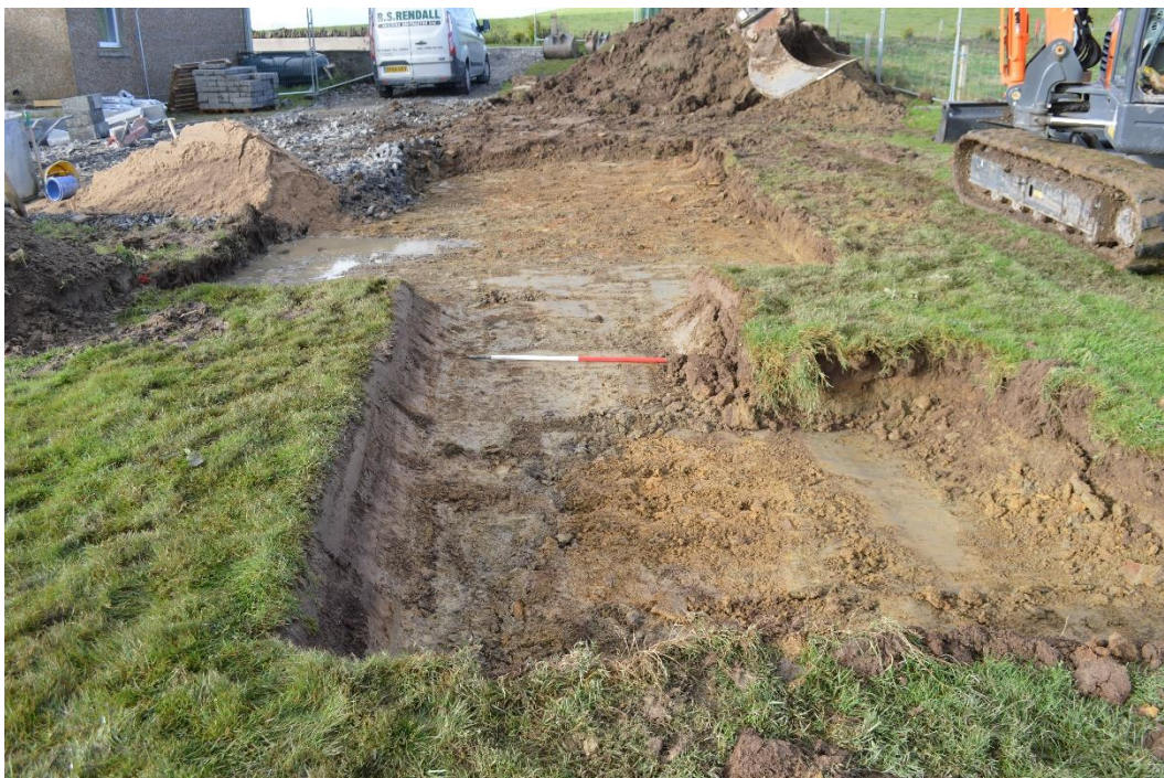
Plate 8: General view, looking west, of the machine-stripped areas for the soakaway and septic tank.
