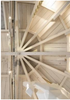
Upper Deck, astern. View of 1820s timber roof reminiscent of Chatham Dockyard slipway roofs (DP 416376, HES, 2023)
