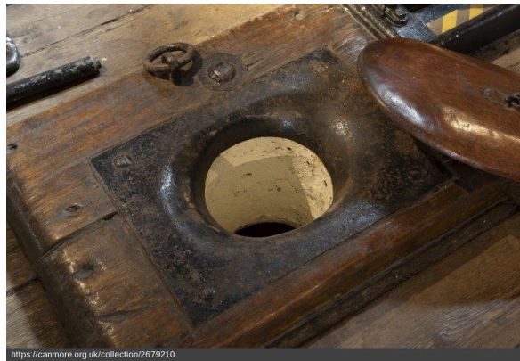
Gun Deck. Detail view of one of two navel/hawse pipes. These fed the capstan chain into the chain locker housed in the Orlop deck (between the Hold and the Lower Deck (DP 416462, HES, 2023)
